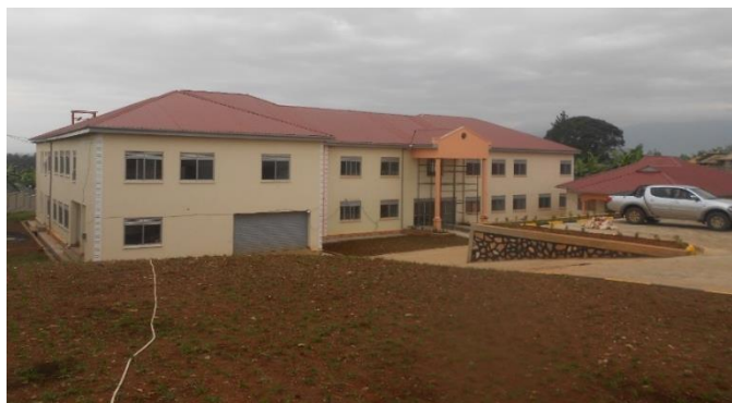
Finishing works on the Minerals Beneficiation Centre at Boma, Fort-Portal City, Kabarole District
