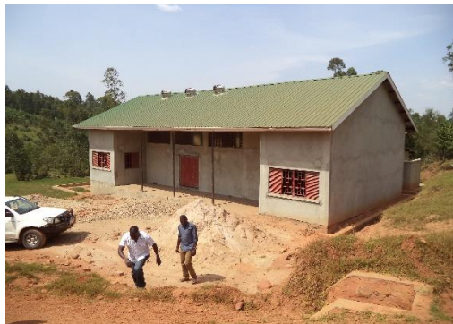
Uncompleted coffee huller shelter in Bushenyi district
