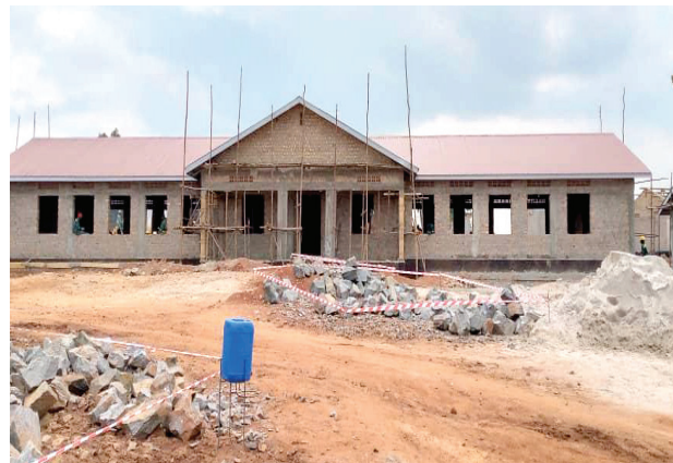
Front View of the Science Laboratory under Construction at Kimenyedde Seed Secondary School, Mukono District
