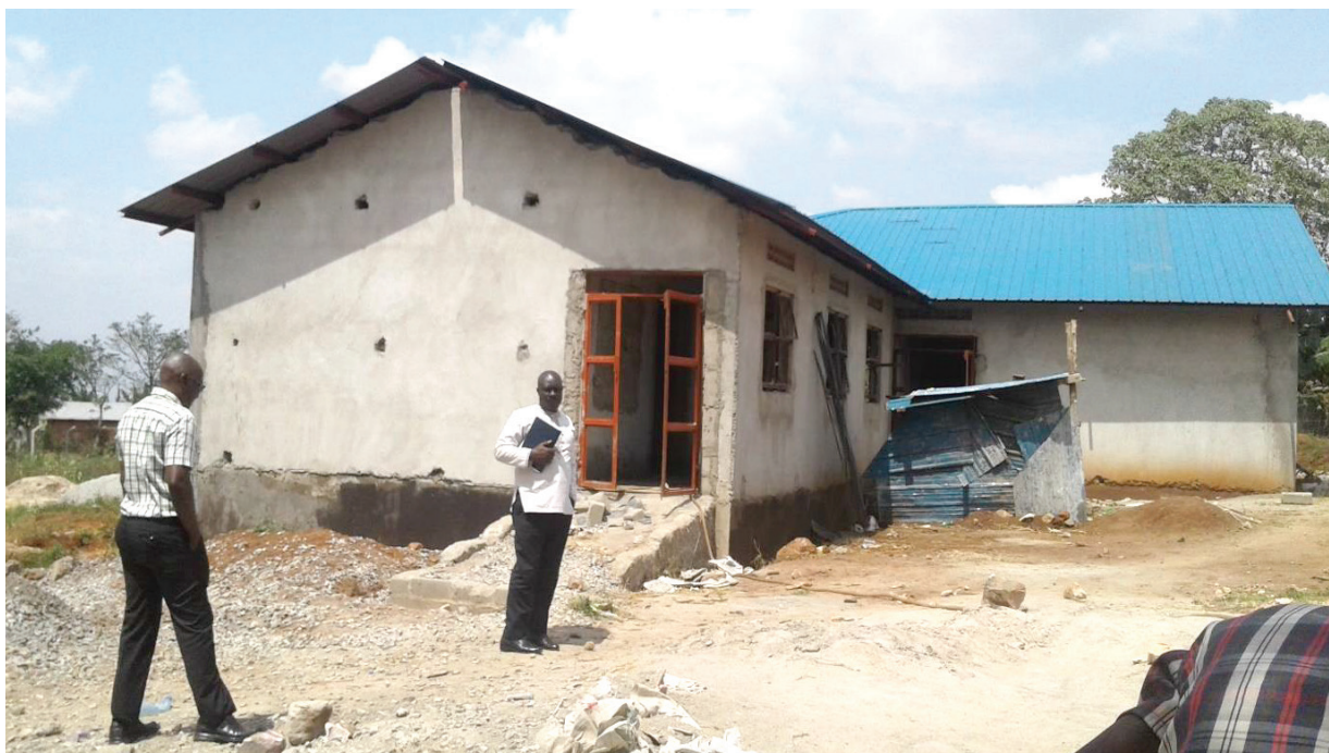
Construction of General Maternity Ward at Bulaga HC III in Kiboga District, Central Uganda showing features of substandard work
