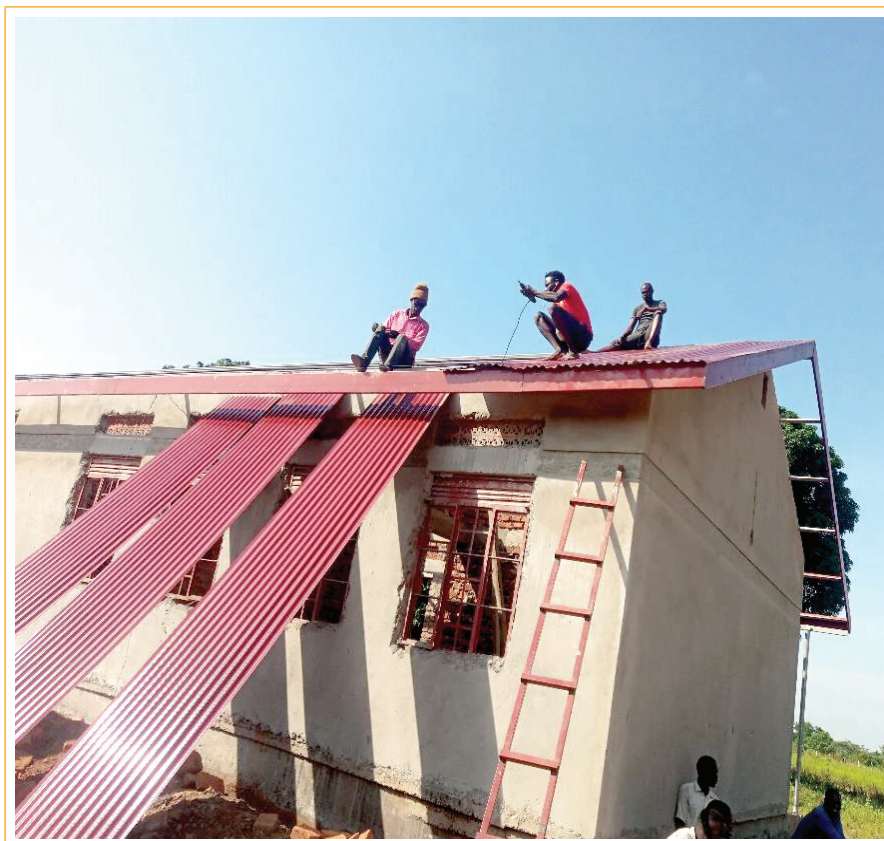
Workers roofing one of the Classroom Blocks at Ngora Seed Secondary, Ngora District, Eastern Uganda without Personal Protective Equipment (PPE)
