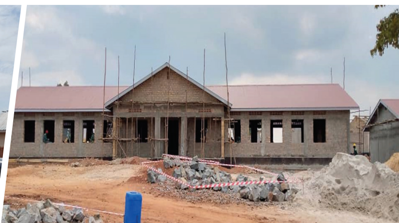
Front View of the Science Laboratory under Construction at Kimenyedde Seed Secondary School, Mukono District
