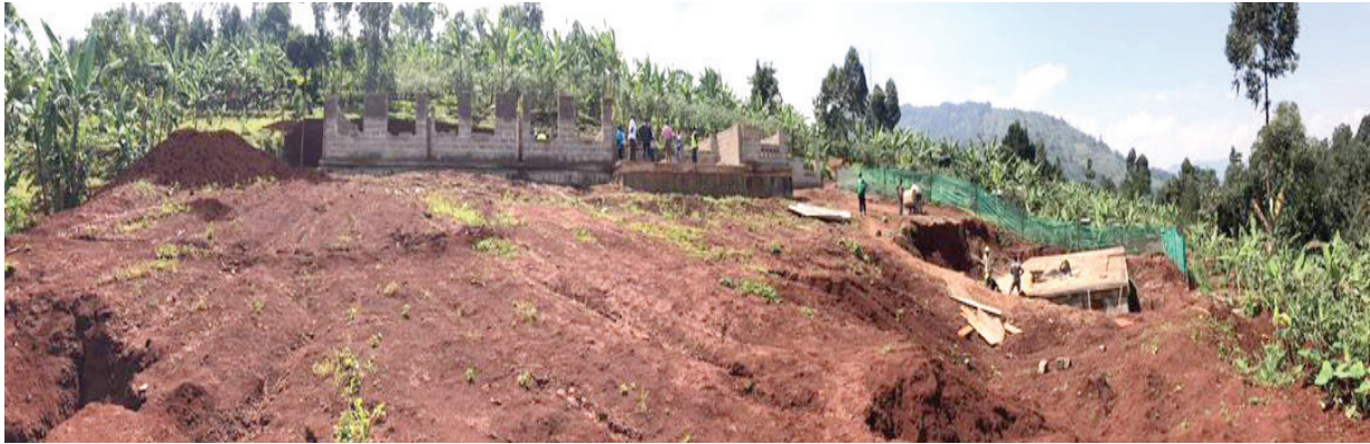
Soil erosion/huge gullies seen on the construction site of Bunamono HC III in Bududa District, Eastern Uganda
