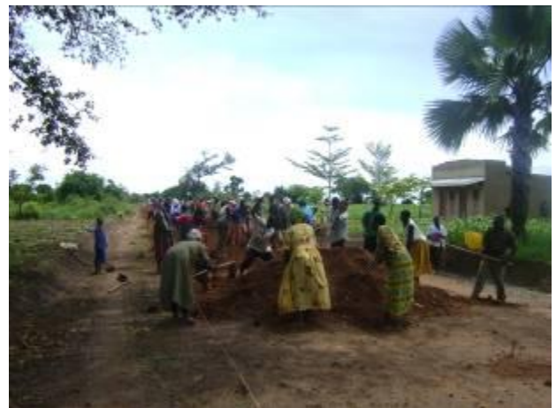
Picture shows re-gravelling of Barr – Apach Br road by labour based contractors in Lira district
