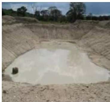
Construction of a valley tank; a shallow well will be constructed using the same water source for domestic consumption, Kiruhura
