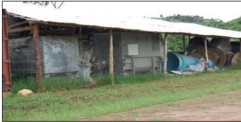
Electrical mechanical equipment under a temporary shelter at Nyagak
