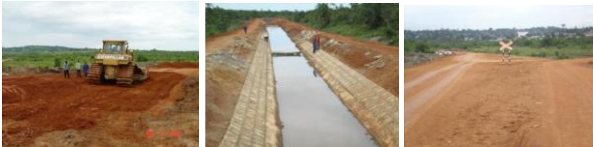
Construction of roads, river slopes and clearing of old Jinja road at a railway crossing
