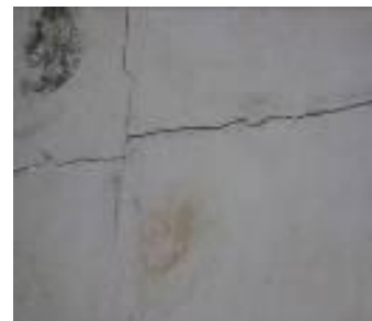
Eminent cracks in the ceiling of BugaboHC3
