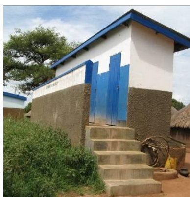
Rehabilitation of ECOSAN with no access for people with disabilities, Amida SC. Kitgum
