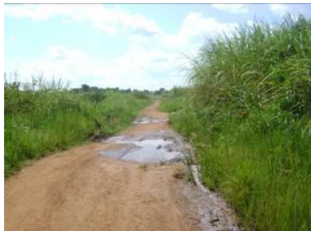
Picture shows a section of Pakanyi – Nyakarongo road in Masindi district where routine maintenance was done
