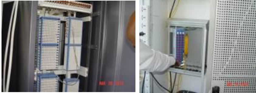
Equipment installed at the Foreign Affairs ministry
