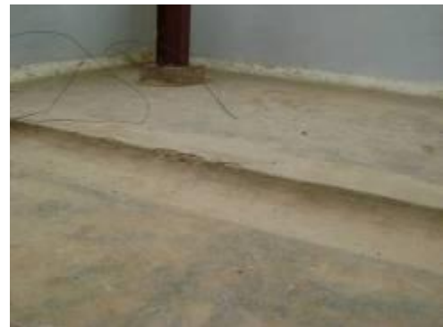
Cracks in floor of slaughter shed
