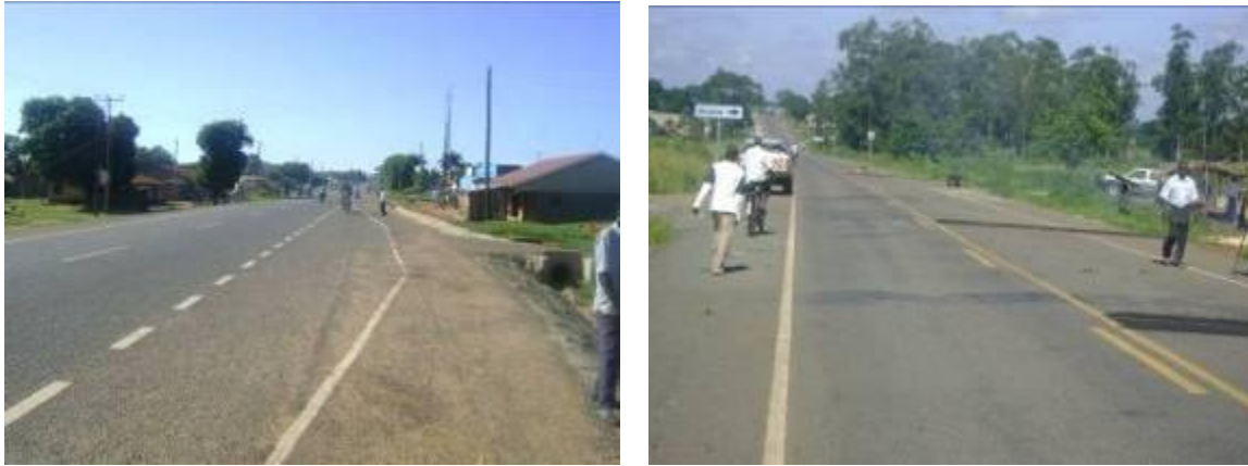
Soroti – Dokolo road: A completed section of the road (Left) and construction of rumble strips at Anyara trading centre (right)
