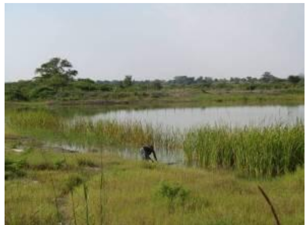
Olamia valley tank in Apac constructed at a unit cost of US$ 34,000 per m 3 . Site is one year delayed and still incomplete; a beneficiary is accessing water directly – a public health risk
