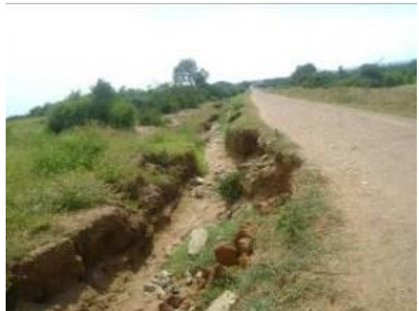
Heavily eroded side drain along Bukumi – Butyaba road
