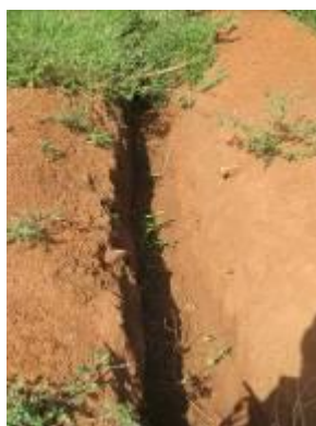
Trenching done but left uncovered posing a health and safety risk, Madi Opei RGC, Lamwo district
