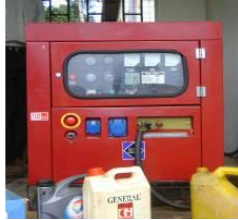
Generator for eye & admin Dep'ts
