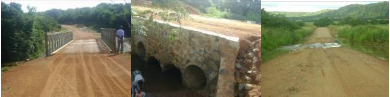
Works done by force account: Wambabya Bridge and the newly alternative crossing at River Rutooha both along Parajwoki – Kaiso road; and one of the water crossings along Sabasolo Landing access link where culverts were required.
