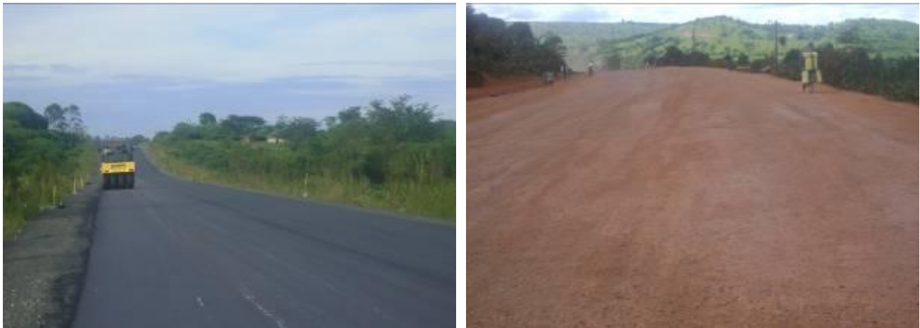
Masaka – Mbarara road: Ongoing works at different stages of completion. Asphalt Surfacing (left) and Earthworks (right)
