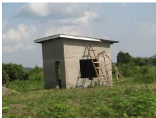
Incomplete construction of the pump house, Ayara RGC, Kole district
