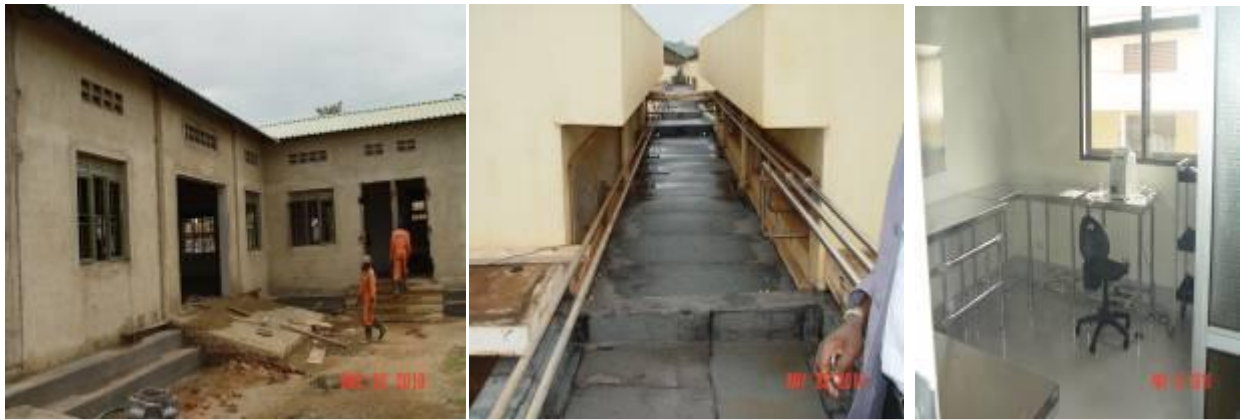
New Gel House, repaired Roof corridor and Newcastle vaccine laboratory at UIRI
