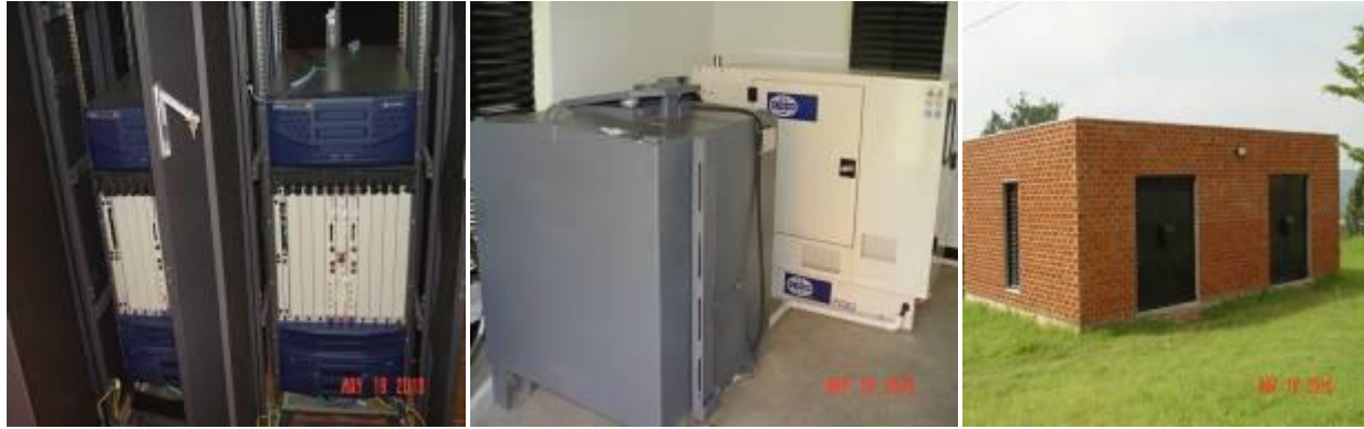
Server racks, Fuel tank and generator, and structure housing the NBI site in Bushenyi
