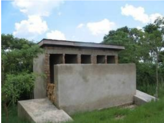
Construction of an ECOSAN facility at Bukalango Prayer Palace in Wakiso district next to a water borne toilet
