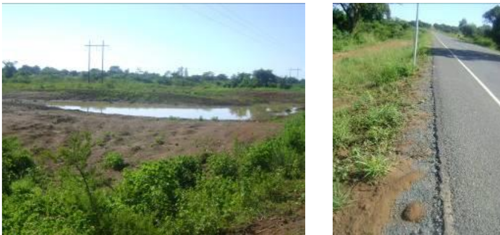
Soroti – Dokolo Road: Water pond at a reinstated gravel borrow pit (left) and a section with defective side slope top soiling and grassing
