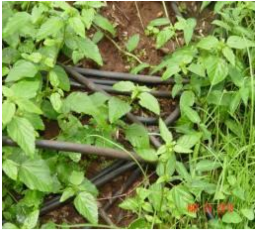
NBI Cables at the Tororo Site
