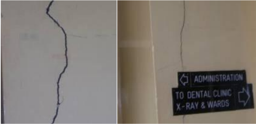
Cracks in the administration building
