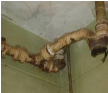
Rusty water pipes to be repainted.
