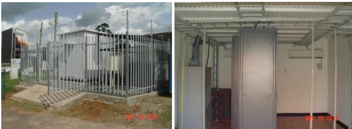
Kabarole NBI facility and mounted racks with equipment
