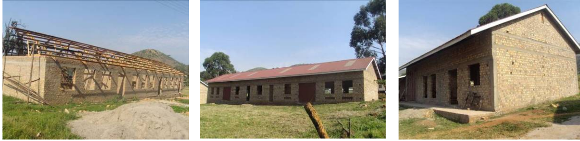
Classroom block at roofing level, a twin workshop (plumbing) and an MV workshop at finishes level.
