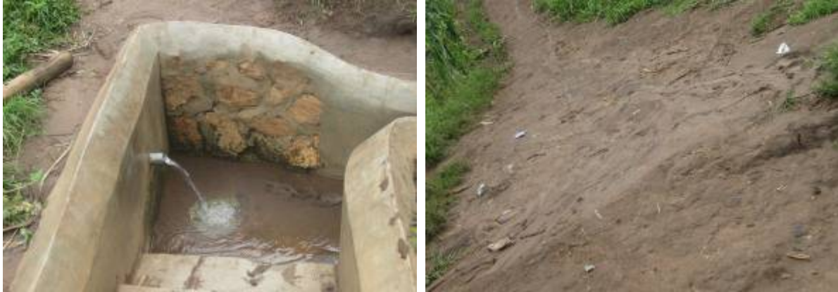
Photos 5&6: Protected spring in Kumi.it is yielding at less than 50% of design capacity due to degradation of the catchment area on the left.(photo taken 21/06/2011
