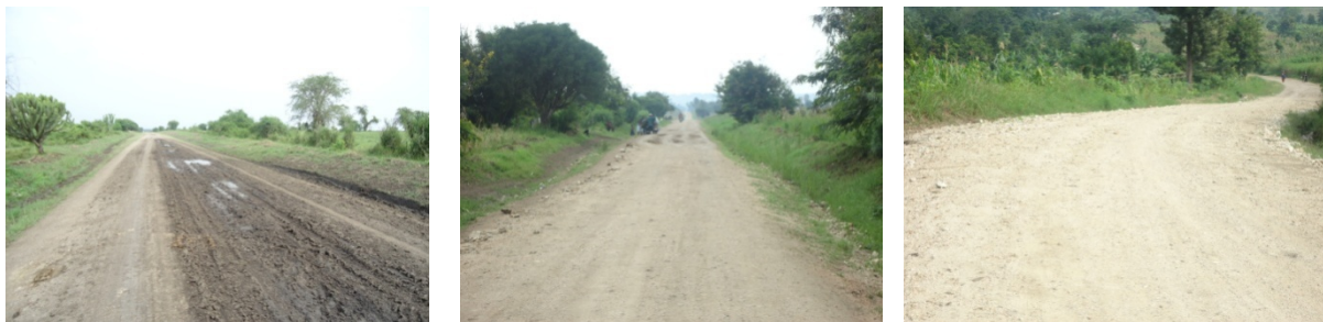
FIGURE 9 LACK OF COMPACTION HAS COMPROMISED THE VALUE OF THE MAINTENANCE INTERVENTIONS ON THIS KATWE – KATOJO – BWERA ROAD
