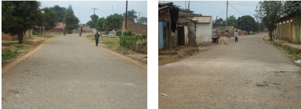
FIGURE 10 A RESEALED SECTION OF MARKET ROAD (LEFT); A RESEALED SECTION OF SEMPIJJA-BULINGO ROAD.(RIGHT) WITH ONE SEAL AND UNPROTECTED SIDE DRAINS.
