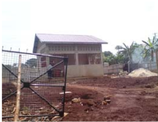
Jinja Regional Referral Hospital: renovated theatre (top left); new incinerator house (top right); works on staff accommodation (bottom left and right)
