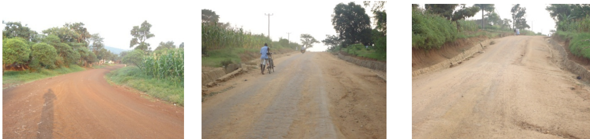
FIGURE 6 GRAVELLED SECTION AT 12+500, GULLEY EROSION AT 20+400 AND ERODED STONE PITCHING AT 20+600
