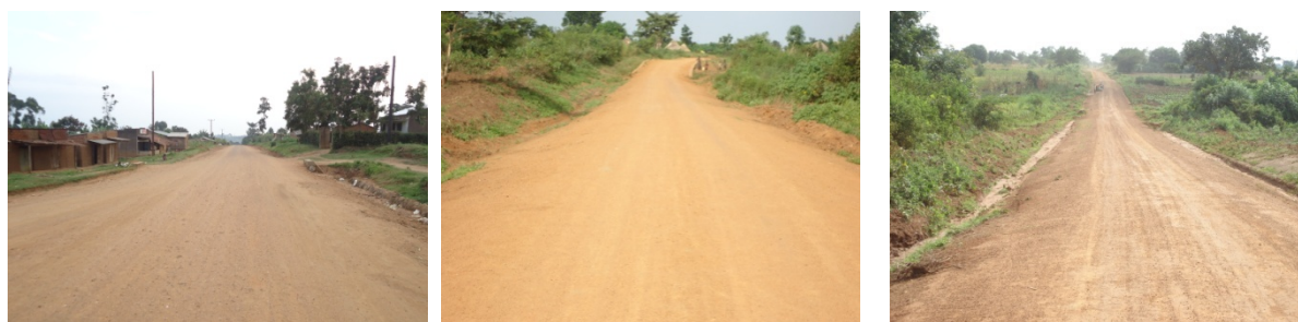
FIGURE 8 ROAD IS EXTREMELY WIDE AT KADOTO (KM 0+000), COMPLETED SECTIONS WITH RAISED CULVERT APPROACHES IN THE BACKGROUND AT KM 25+800 AND 31+800
