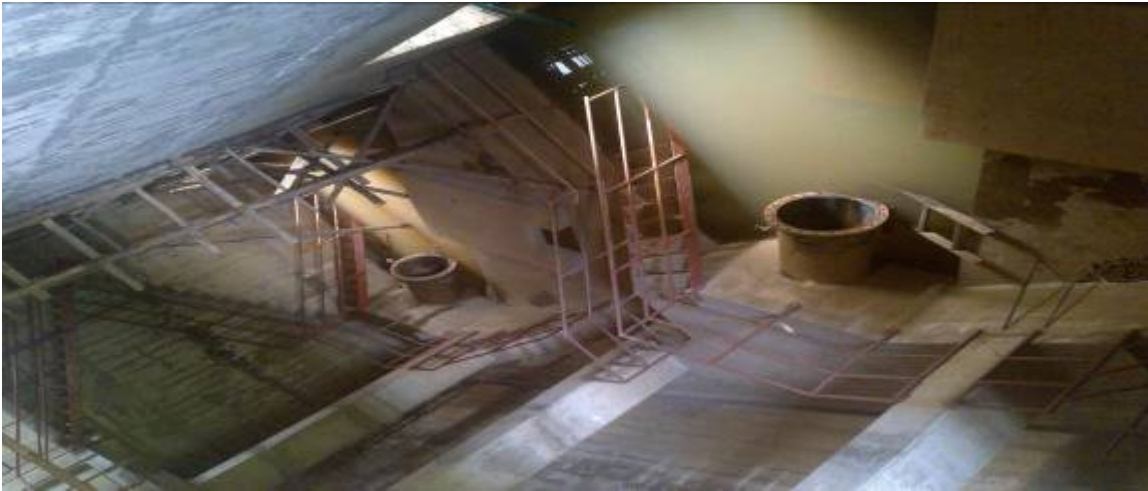
Power house awaiting installation of Electro Mechanical Equipment
