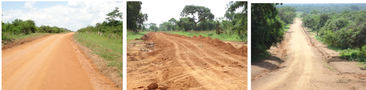
FIGURE 1 COMPLETED GRAVEL WORKS AT 25+200, DUMPING AND SPREADING OF GRAVEL AT 27+000 AND GRADED SECTION AT 29+500
