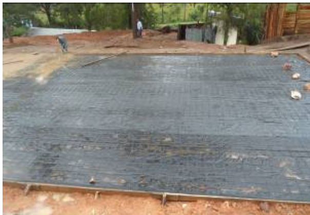
ICT lab at substructure level- Kinyasano Girls
