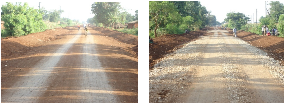
FIGURE 7 GRADING TO THE REQUIRED SLOPE ALONG MUYEMBE-NAMALU ROAD AND APPLYING OF STONE AGGREGATE ALONG MUYEMBE- NAMALU ROAD SO AS TO ACHIEVE A FIRM SURFACE.
