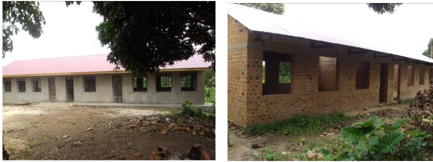
A 2-classroom block with an office and another 2 classroom block at finishes level
