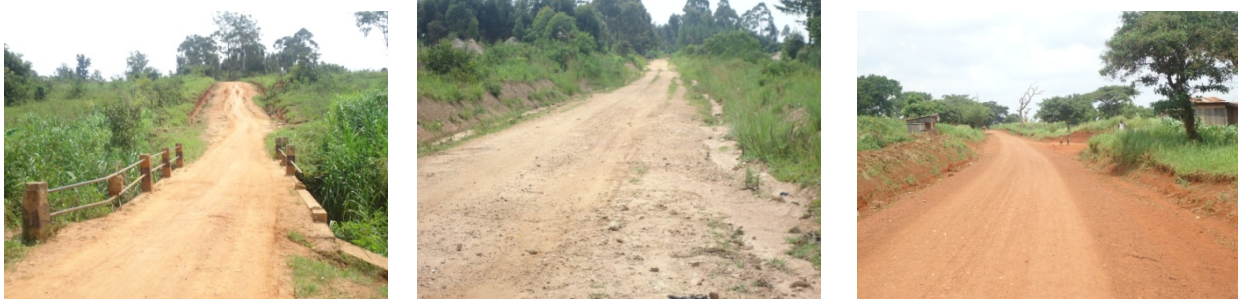
FIGURE 3 AYAVU BRIDGE AT 0+000, POORLY CONSTRUCTED SECTION AT 2+700 AND COMPLETED GRAVEL SECTION AT 25+300
