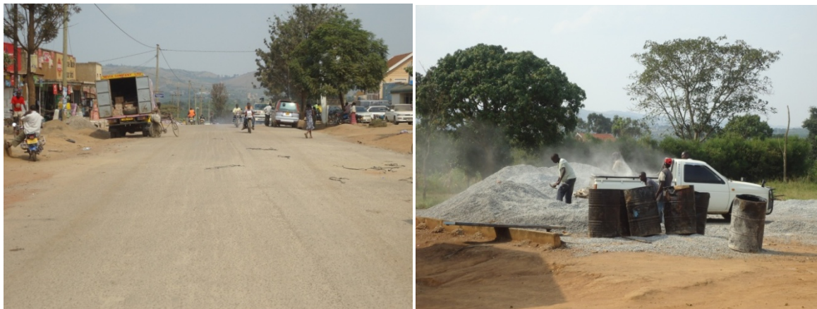
FIGURE 11.1A RESEALED SECTION OF MARKET STREET WITH THE SECOND BITUMINOUS LAYER (LEFT); ADDITIONAL CHIP STONE AND BITUMEN WAS ALSO SEEN AT THE TOWN COUNCIL YARD
