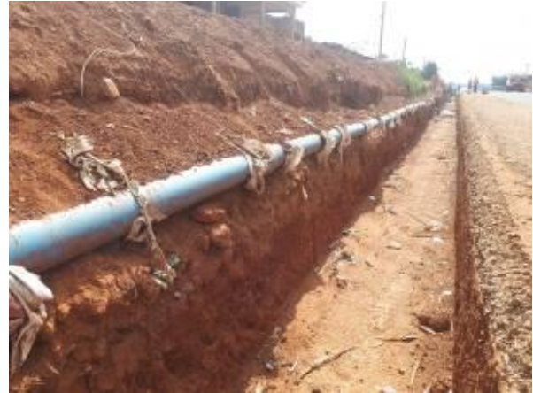
Musita Lumino: A water distribution line in the right of way of the road
