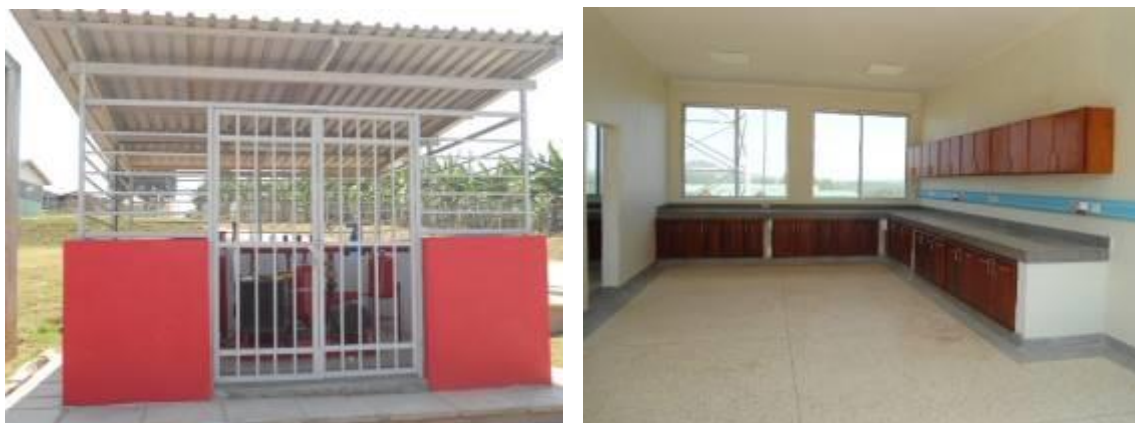
Installed Firefighting Unit and a furnished laboratory in the Quality assurance block at the TBI in Bushenyi
