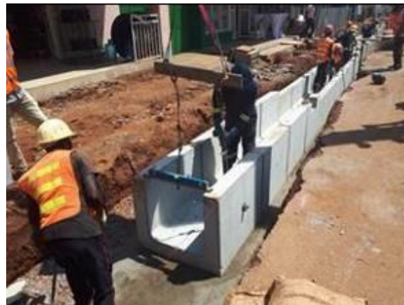
Placing U-drains on one of the roads in Gulu municipality Under JICA
