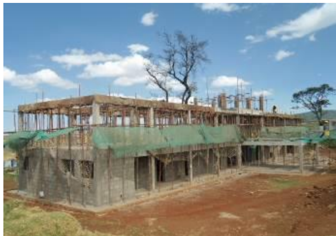
The hostel block at the National High Altitude Training Centre at Teryet in Kapchorwa District
