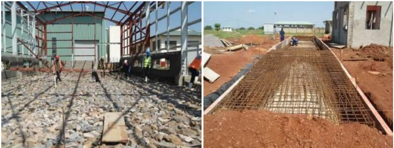
Ongoing construction works at CDO cotton seed dressing station in Pader District
