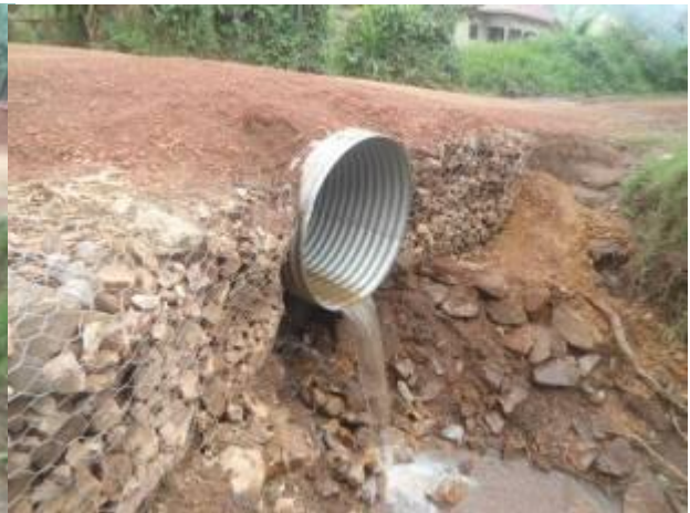
Emergency works of a 900mm diameter armco culvert along Sindi-Mparo road at km 1+100
