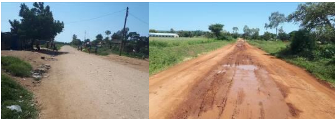
A section of Wandu-Rhino camp (51km) in good condition by virtue of term maintenance in FY2017/18 A gravelled section of Wandu-Rhino camp that had deteriorated following heavy rains
