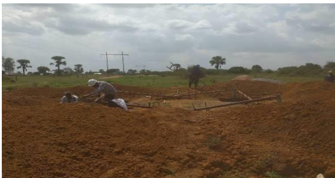
On-going Tower foundation works at Soroti Airfield, works at this location area as a result of transmission line diversion at Soroti Airfield
