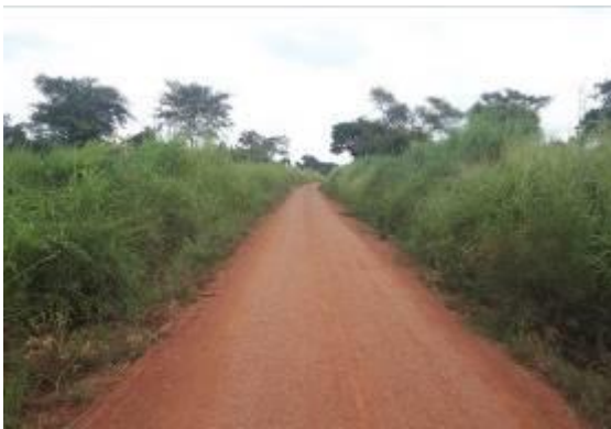
Grading and spot gravelling on Labora-Loya-Ajonga road(29.9km) was done in Q3 FY2017/18 but no routine manual maintenance
