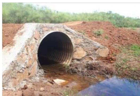
Single cell 120mm Armco culvert installed at the swamp section on Nsinze-Naigobwa Road
