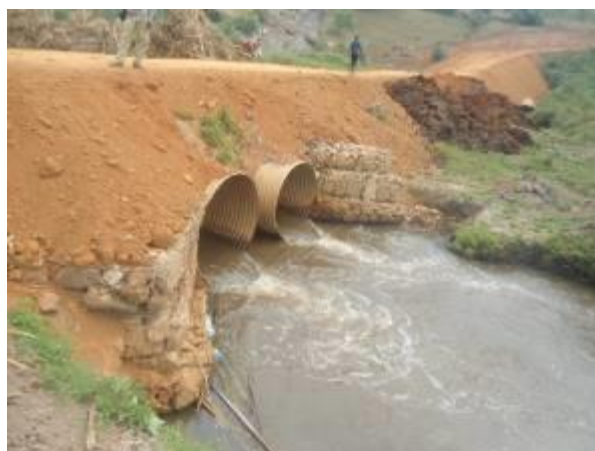
Nyakibobo-Buhanama-Rwentoyo (12km) in Ntungamo: Ongoing swamp filling works and installed culverts at km 7+000
