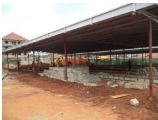
Works on Bulk Agricultural Delivery and Auction Centre and Shelters for Matooke in progress at Nyendo Market
