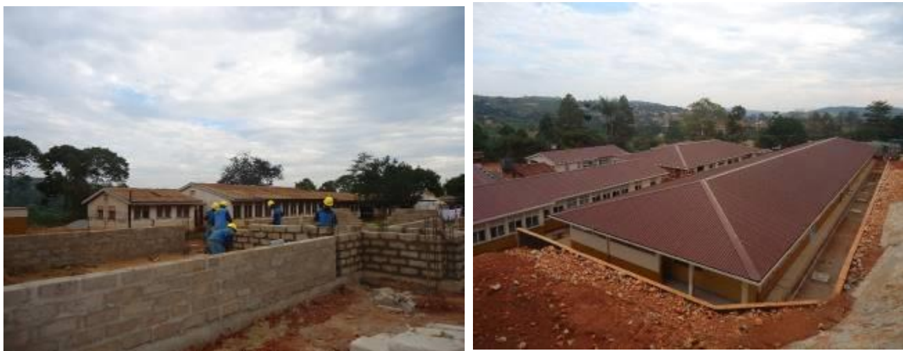
L-R: Ongoing construction works; Some of the completed structures at Kawolo Hospital in Buikwe District
