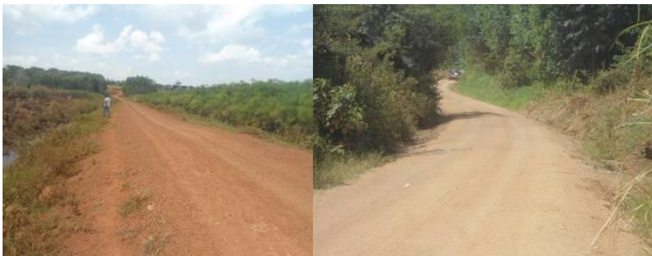
A raised section of a swamp on Kagavu-Nabakazi-Kikandwa road between km 7+200 and km 8+400
