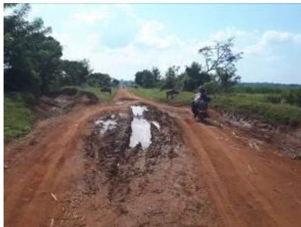
Kamuli-Namasagali road; the sandy nature of the soils facilitates quick wash outs during the rainy season
