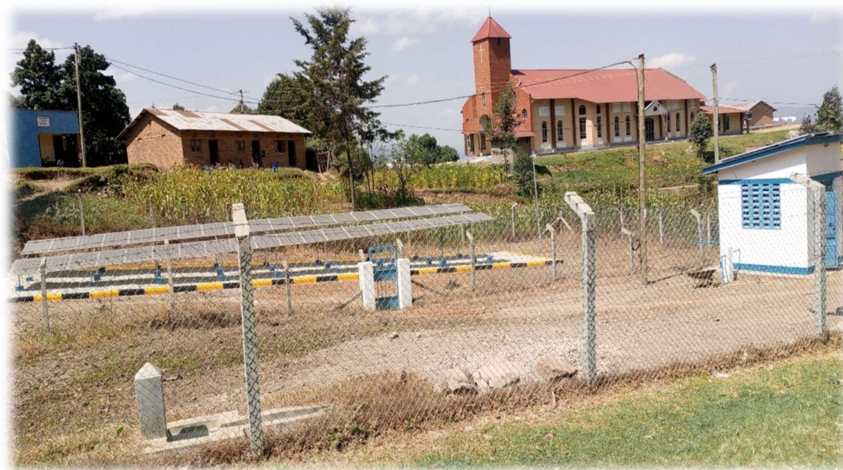
Solar panels installed and connected to the pump house at Burime Primary School
