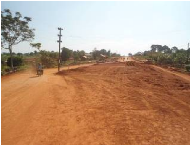
REA electricity poles in the middle of the project road at Km 21+600 on Misuta–Lumino road
