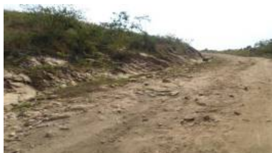
Rocky section along Minera–Nyabushenyi road with very loose material
