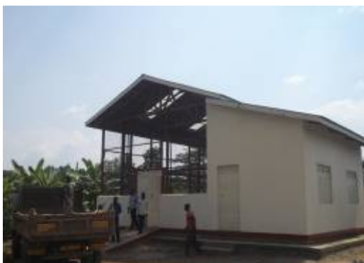
Ongoing construction of an abattoir at Nagongera Town Council in Tororo district by 13th August 2016
