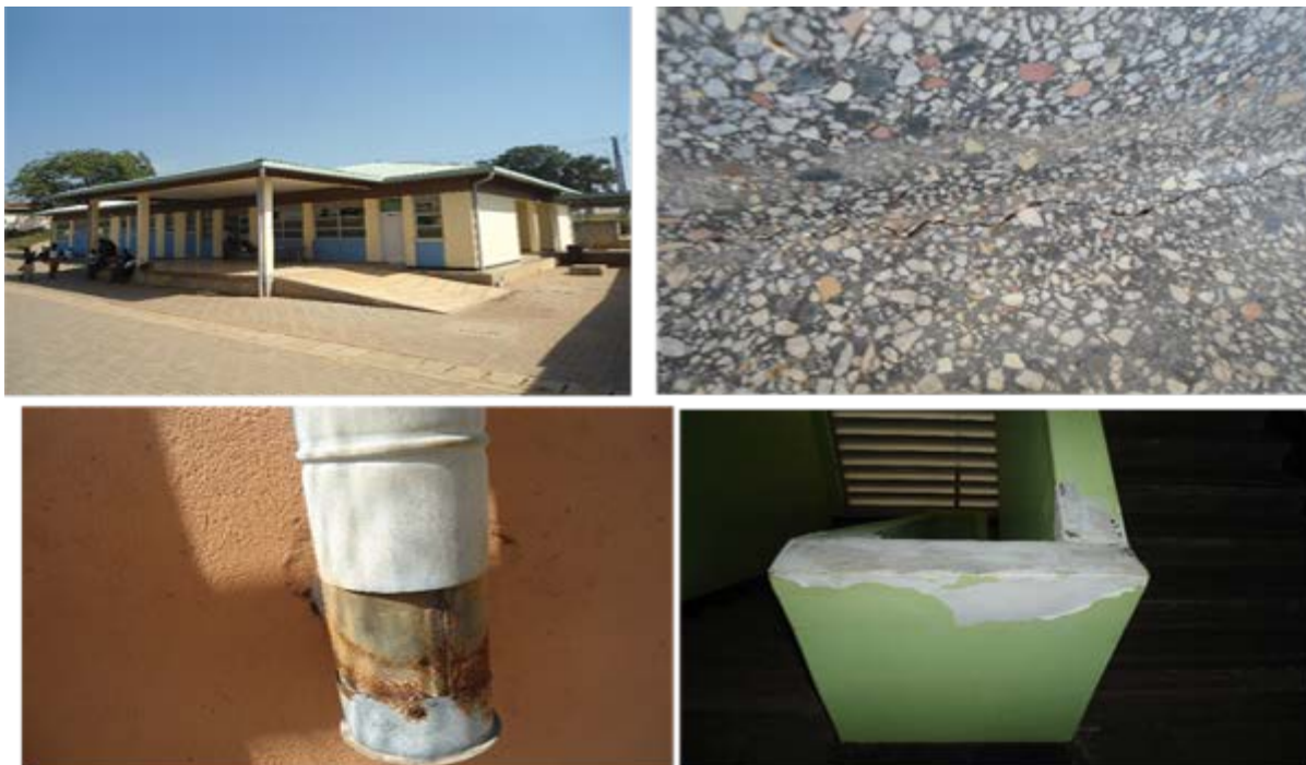
Left: Causality infrastructure at the Three million dollar project at Nebbi Hospital Right: Cracks in the floor, rusting Chimney at the attendants kitchen and paint peeling paint in some of the T-block at the same hospital
