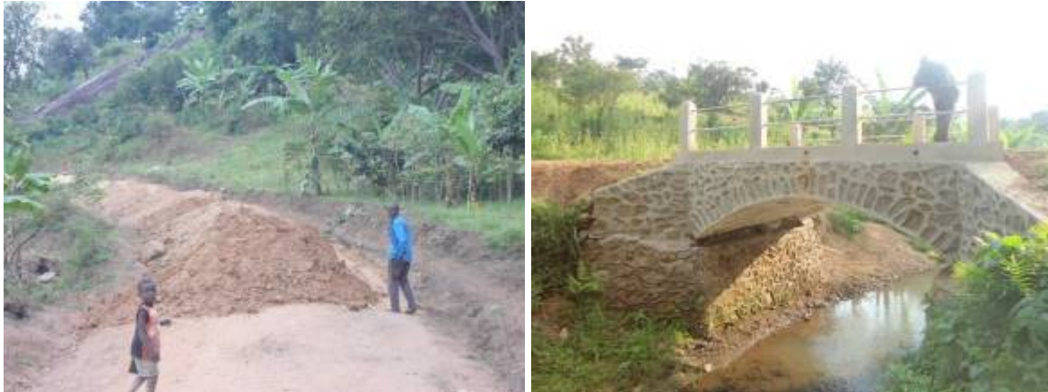
Left: Dumped material along Nabweye-Bukikali road in Lwaso Sub-county for the gravelling activity; Right: A stone masonry arch bridge across River Wangoko on Nanyuna-Mukosi road at km 3+400 in Nyanyusa Parish in Mbale district
