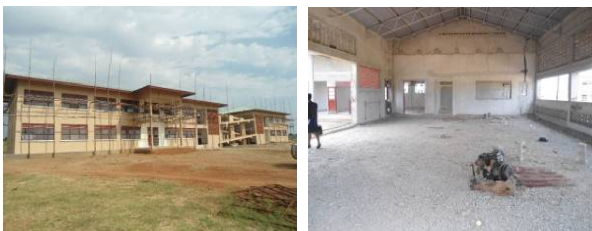
Left: The incomplete administrative complex Right: Inside the incomplete workshop complex at Bukedea T/I. Ms Togo construction complex abandoned this site without completing all works complaining of non-payment.
