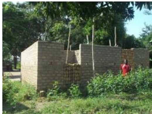
Mr. Ogwan Nixon's permanent house constructed out of cotton sales in Lakwana Sub-County, Omoro district
