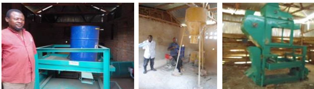
L-R: Parts of the coffee grader delivered to Kololo Progressive farmers, a maize mill at Tukolerewamu both in Mpigi and installed coffee processor in Busongora-Kasese
