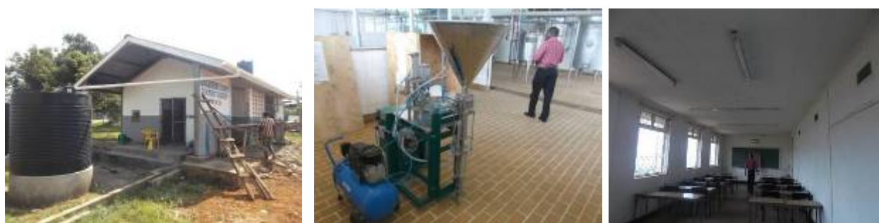
L-R: Bbaale Milk Collection Centre undergoing rehabilitation in Bbaale sub-county Kayunga district; Yorghut making machine and rehabilitated ceiling in administration block at Entebbe Dairy School in Vet village Entebbe Municipality, Wakiso district
