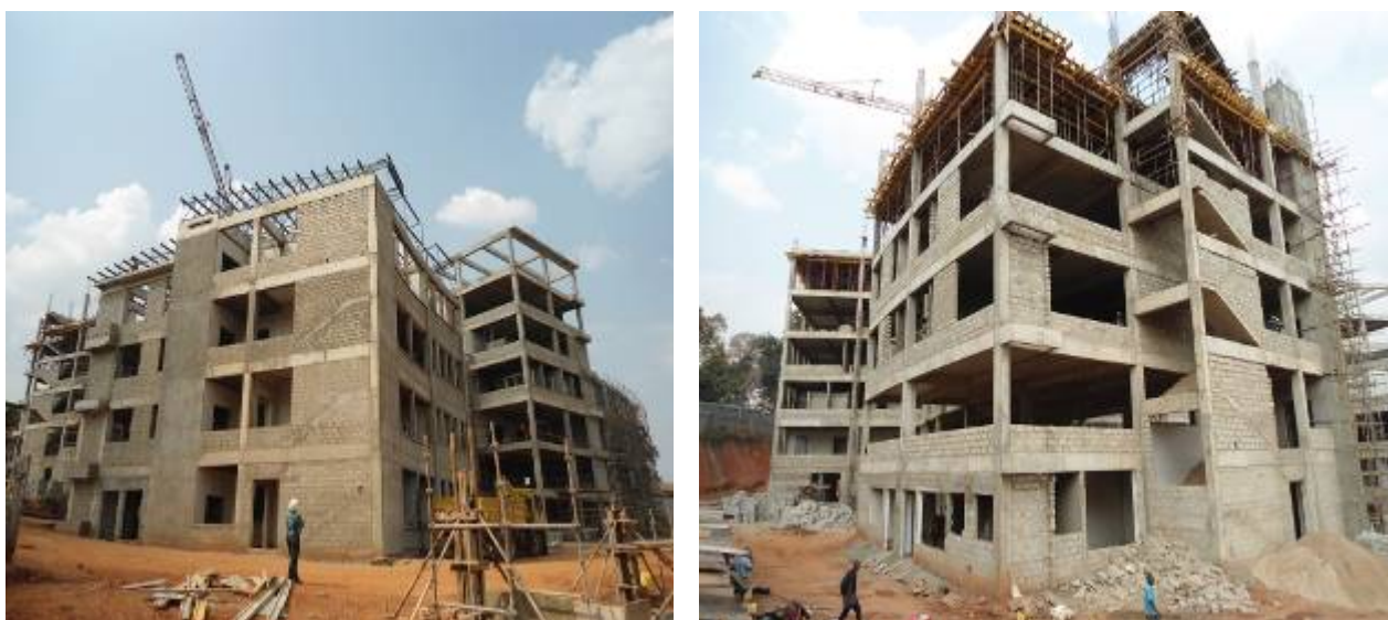
Different views of the construction works at the neonatal and maternal unit
