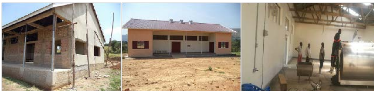
Left: Incomplete APFMilk cooler facility in Shuuku sub-county, Sheema district; middle: Completed APF in Rukiri sub-county, Ibanda district but non functional; right: installation of a Milk cooler in Rugarama sub-county, Ntungamo District
