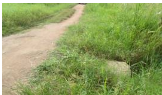
Poorly maintained road with an incomplete culvert line at km 5+200 along Kasenyi-Nyakabingo
