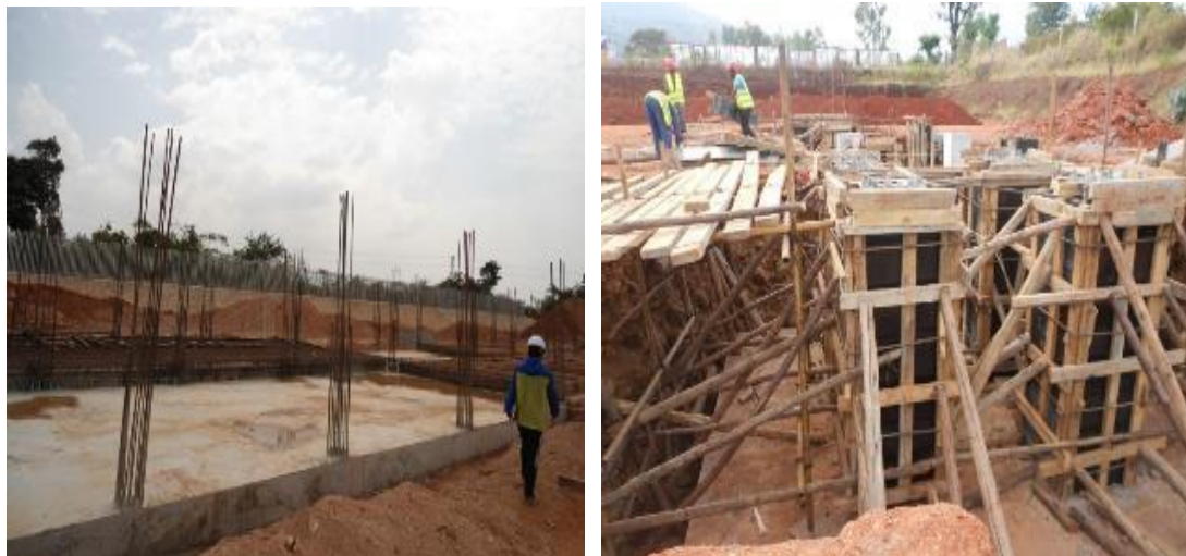
L-R: Foundation works for the plant house in Hoima substation; Civil works for equipment and overhead gantry foundations at Nkenda substation
