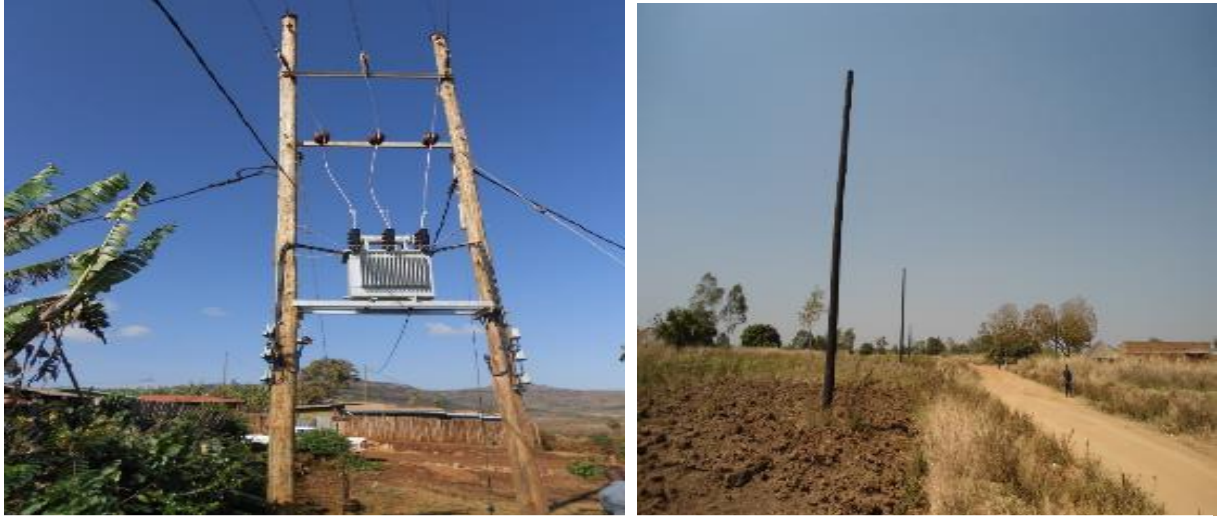
L-R: Installed transformer on the completed 33kV Kapchorwa-Bukwo-Suam line, Poles erected on the Ociba Community share scheme in Arua district
