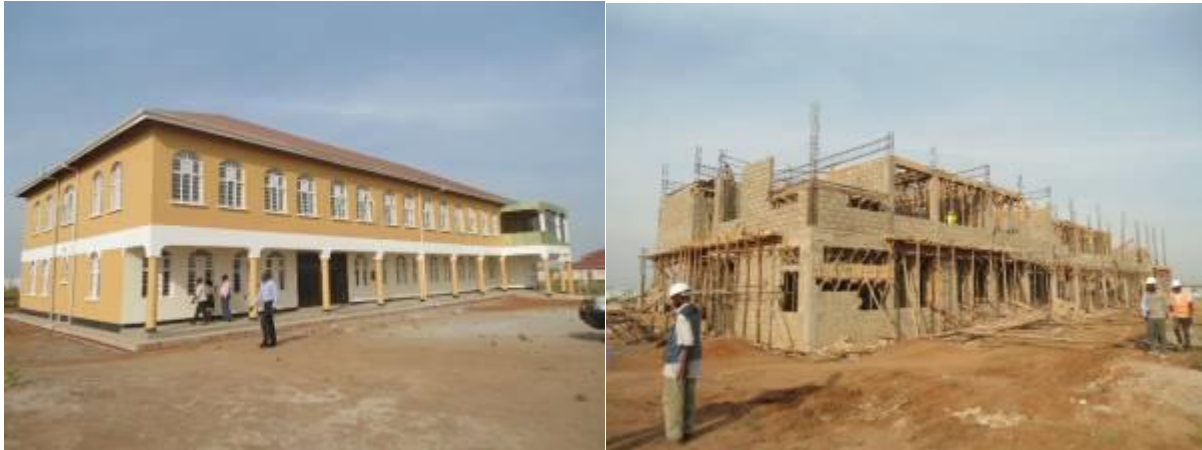
L-R: The completed Public Health block, and the Health Sciences block under construction at Lira University
