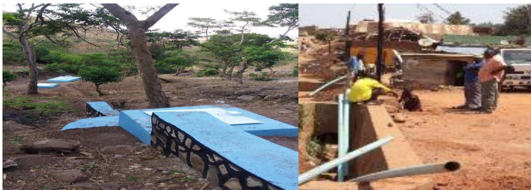
L-R: Protected water catchment at Murema water source; Community members excavating water trenches and laying pipes for the water source at Kashumba sub-county, in Isingiro district
