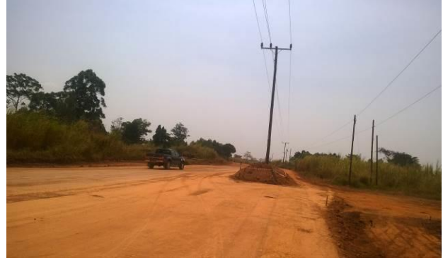
Power lines within the road prism yet to be relocated along the Kabwoya-Kyenjojo road
