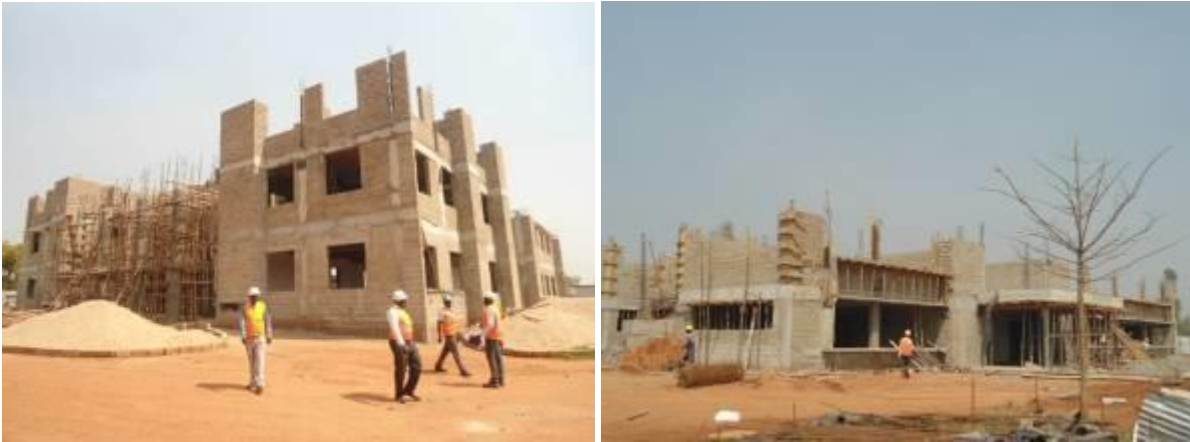
L-R: The agricultural block at 45% and multi-functional laboratory block at 29% progress at Gulu University
