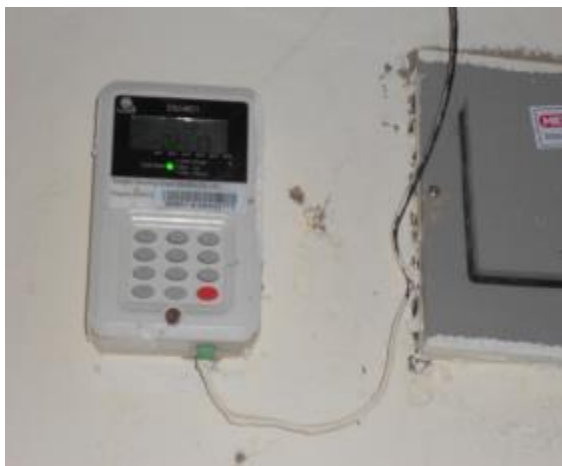
User interface unit on one of the OBA connections made by Kyegegwa Rural Electricity Cooperative Society in Kyegegwa district
