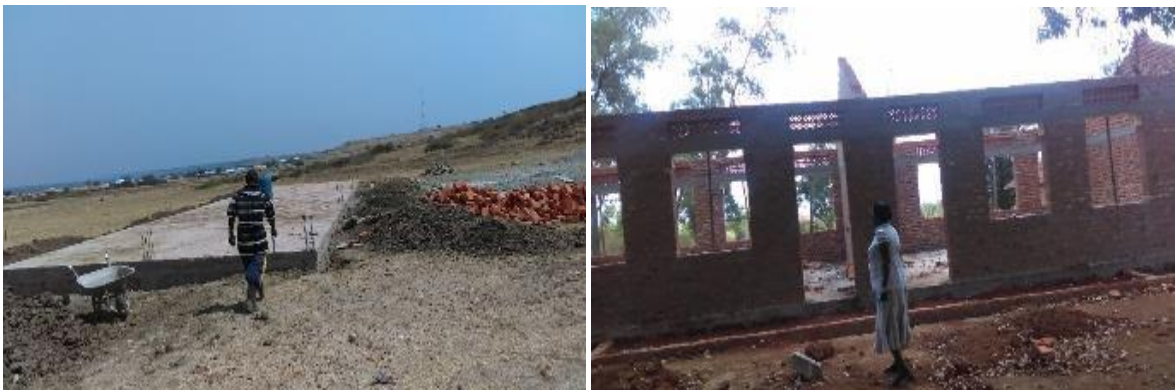
L-R: Foundation works for construction of a two classroom block at Nyawaiga P/S, Hoima; Construction works of a two classroom block at roofing level at Kiriyaadongo CoU P/S Kigumba
