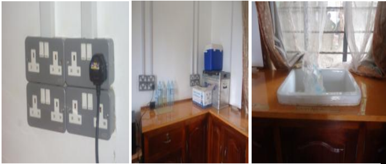
L-R: Industrial sockets; Water samples in bottles, a Cooler, and Microbiological testing kit; Wash area (sink) without water supply installed in the laboratory at Albert Water Management Zone in Kabarole district
