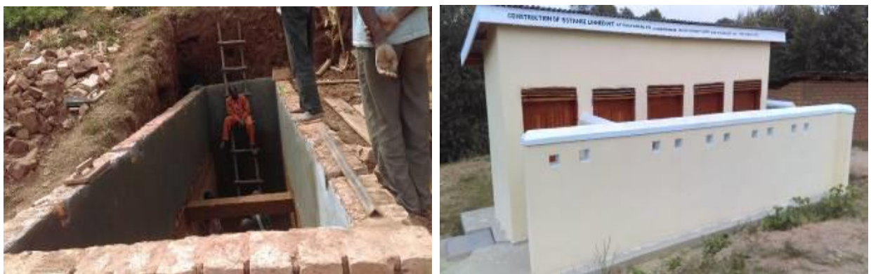
L-R: A 5-stance lined pit latrine under construction at Katuna P/S; Kabale District; Completed 5 stance lined pit latrine at Rwatabaire P/S; Ishongororo Subcounty; Ibanda District.
