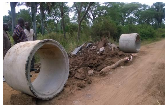
Culvert installation works ongoing along Karugutu – Ntoroko road spilled to quarter three
