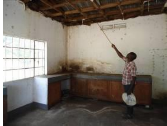
Dilapidated office and laboratory block under use at Nshaara Ranch in Nyakashita Parish, Kiruhura district. Staff were demotivated working from these structures
