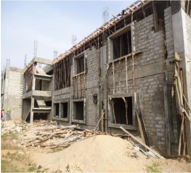
On-going construction works for the Paediatric and Maternity ward at Masaka RRH
