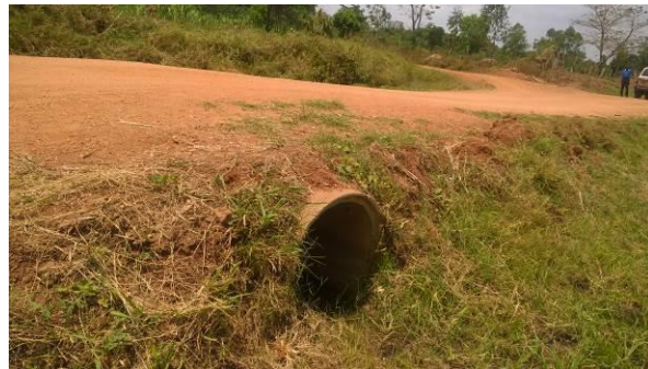
An old culvert installed in the previous years but without head walls
