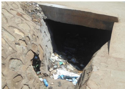
Blocked newly constructed drainage channel in Mbale town along Nakalama-Tirinyi-Mbale Road
