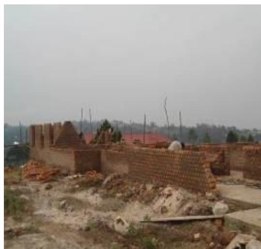
Ongoing construction of the Production Department Office Block at Kunywa Village, Mityana Municipality using PMG funds
