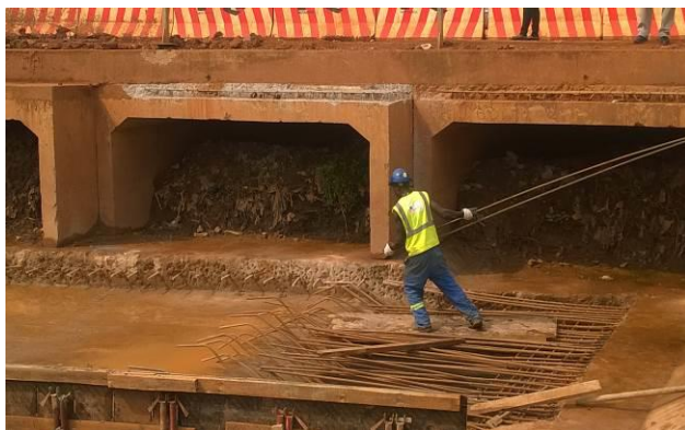
A newly constructed clogged box culvert supposed to discharge water into Lubigi channel, Northern Bypass
