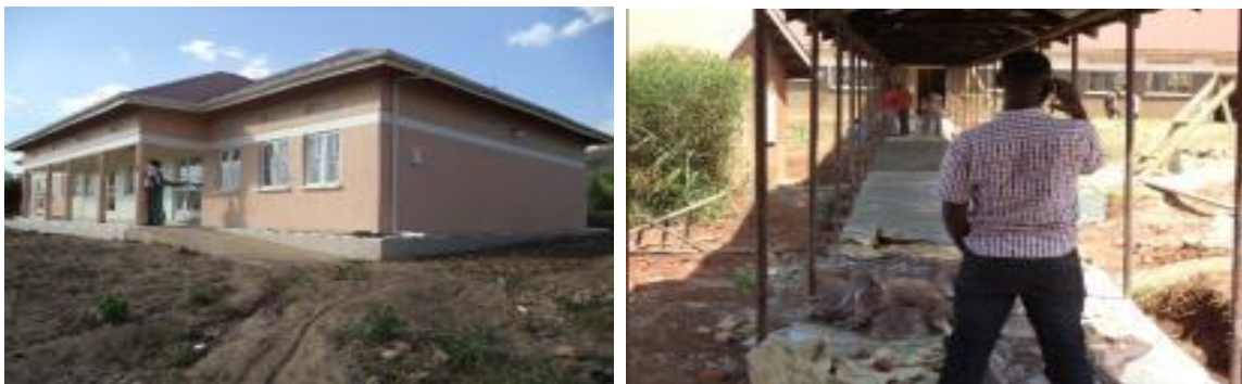
L-R: New Kikagate HC III OPD in Kikagate sub-county; Ongoing construction works on the walkway at Rwekubo HC IV in Isingiro Town Council, Isingiro district
