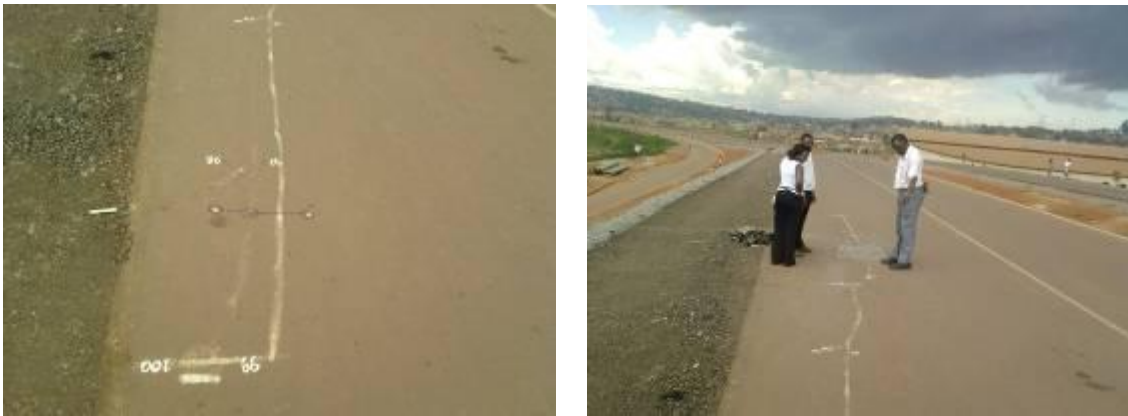
BMAU officers inspecting cracks observed on the approaches to the bridge at Bwaise
