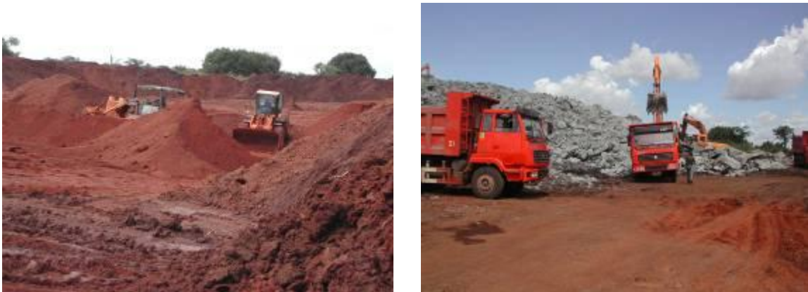
Photos show earthworks and stone quarry works that were in progress during the site visit
