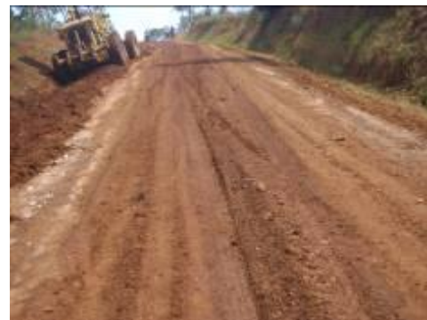
Villa Maria – Kyamulibwa: grading of the road in progress by force account
