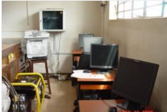
Installed equipment in a small area at Mukono Post Office
