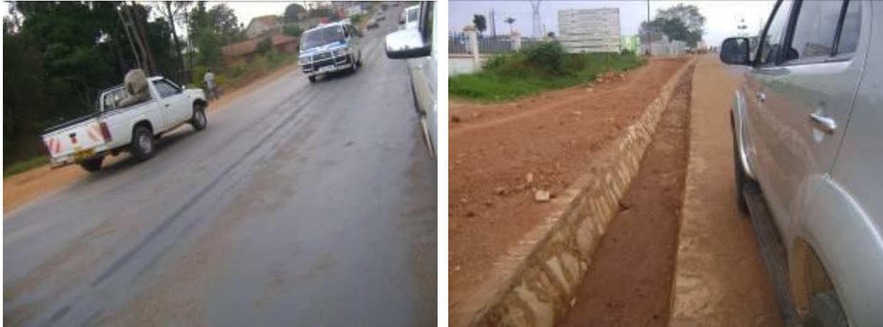
Kampala – Mukono road: A defective resealed section with excessive bleeding (left) and a new stone lined drain (right)
