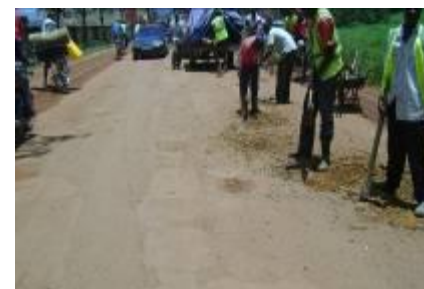
Kabale town roads: Pothole patching in progress but highly ineffective without a drainage system in place
