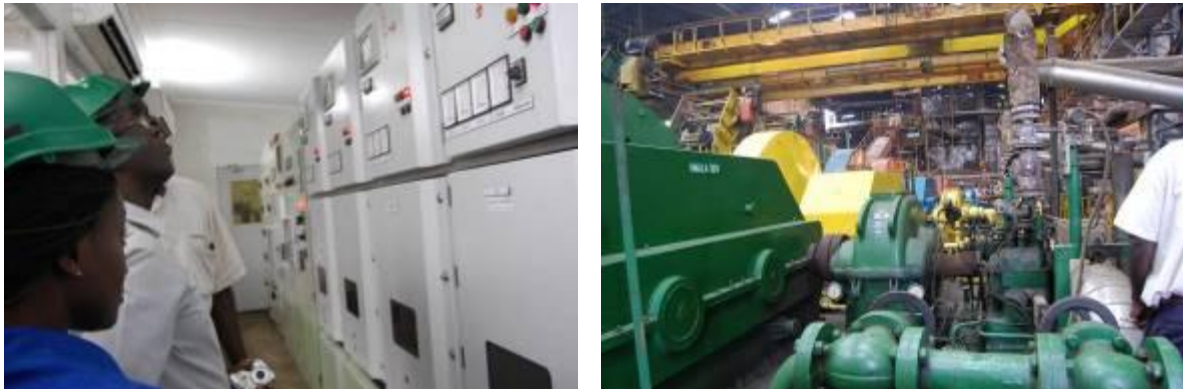
Electromechanical equipment in Kinyara Sugar Limited
