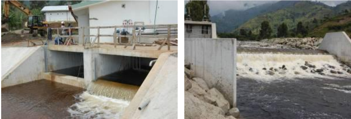
Completion of Civil Works at Bugoye HEP on the Tail Race and Dam/Wier (intake)
