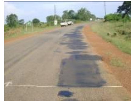
Soroti – Kumi road: section heavily patched on one side of the road showing differential loading on the road.
