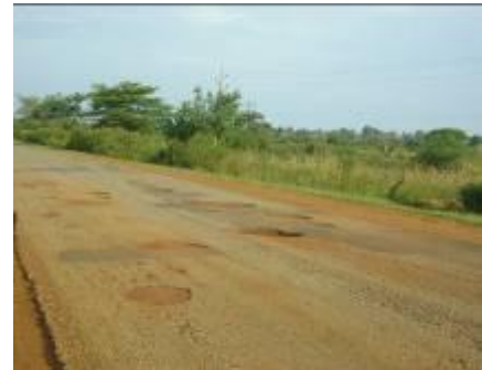
Mbale (Namunsi) – Kumi road: Heavily distressed section with temporary gravel patches
