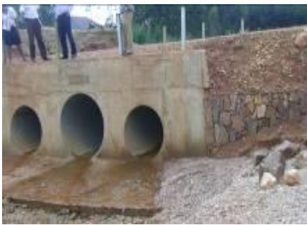
New Rwamwire Bridge on tin quarry access road, off Ntungamo – Kakitumba road.
