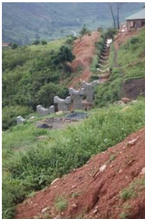
Penstock Anchors at Ishasha HEP
