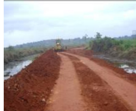
Kyapa – Kasensero road: swamp filling along a 1.2Km swamp done by contract
