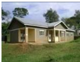
Maternity ward out of use at Kibalinga HCIV
