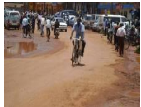
Kabale town roads: Failed drainage system that characterizes the road.
