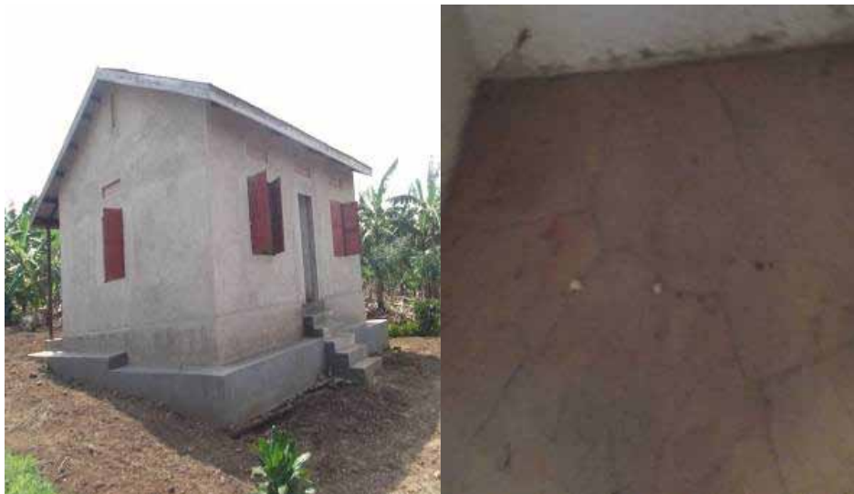
Left to right; resettlement house and cracked floor of resettlement houses constructed by Lamba investments that abandoned site on the Mbarara-Nkenda transmission line
