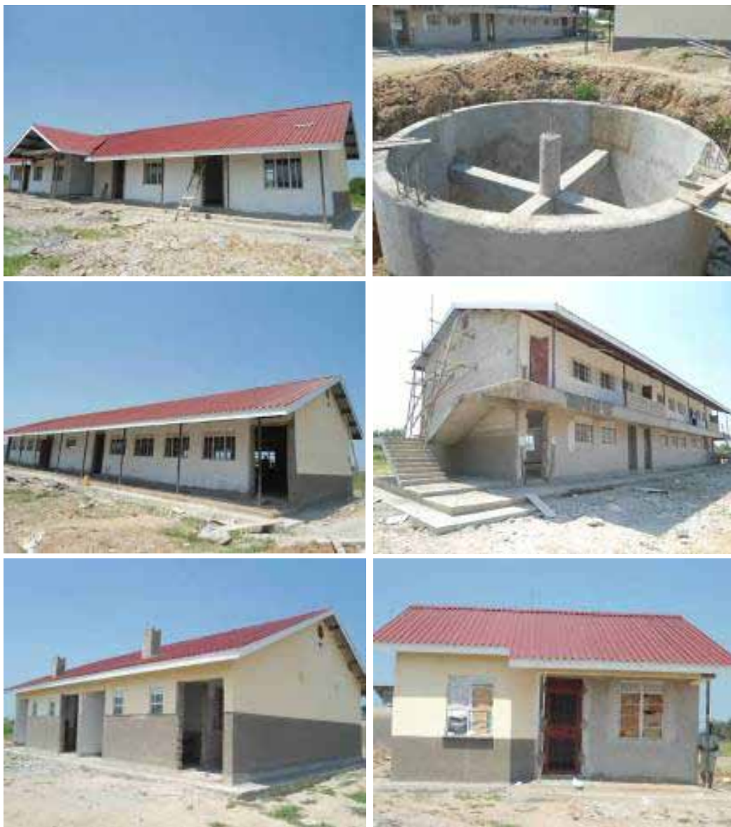
From top left the administration block at finishes level, the under ground tank, a 2 unit science laboratory at finishes level, From bottom left: a storied 6 classroom block at finishes, a 4 unit staff house and a 2 bed room house at finishes level at Kanara Seed S.S The other structures were also at finishes level.
