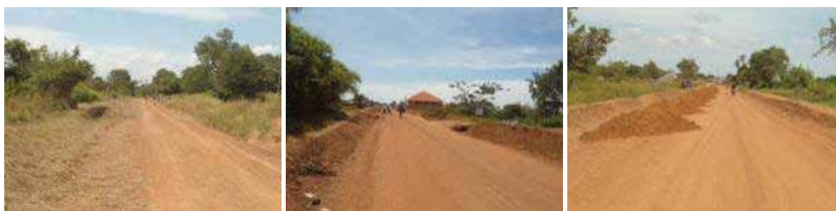
(Left): Well graded section at Km 2+000 with LBC works ongoing; (Centre); A graded section the Km 0+000 from Soroti town; (Right) Murrum heaps for spot regravelling activities at Km 4+500.
