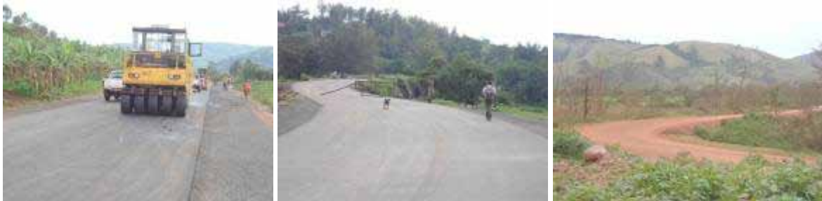
(Left): 50mm of Asphalt Concrete on carriageway and surface dressed shoulders at Km 58+200; (Centre): Completed section without road markings at the end of project road at Murongo Bridge on the border of Uganda and Tanzania; (Right): A section of the 7 Km loop finished with G15 material.
