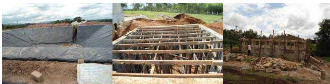
Fertigation house pending roofing, lined water reservoir both at Nyaruzinga, and clarifier chamber under construction at Bumbaire
