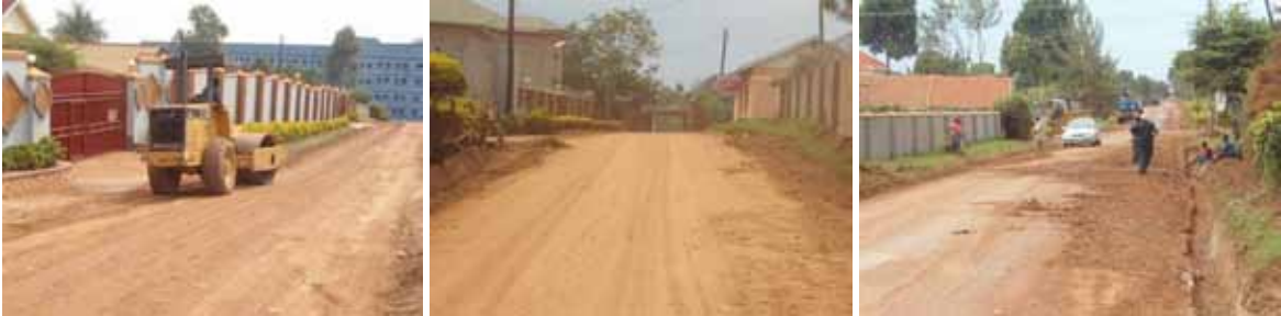
(Left): Compaction of base course works on Alice Reef road; (Centre); Compacted base course on Alice Reef close; (Right): Preparation of lime stabilized material for base course works on Bugonga road.
