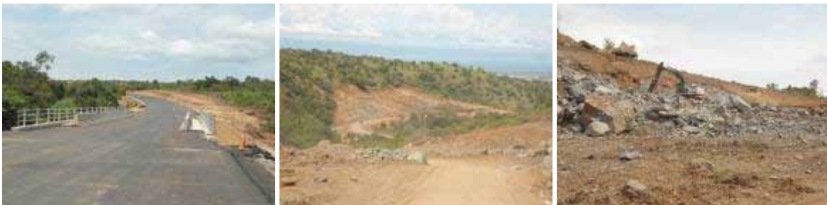
(Left): Completed Wababya Bridge with walkways at Km 34+000; (Centre): New alignment of the road at Km 59+480 with a 28m fill; (Right): Rock excavation along the escarpment.
