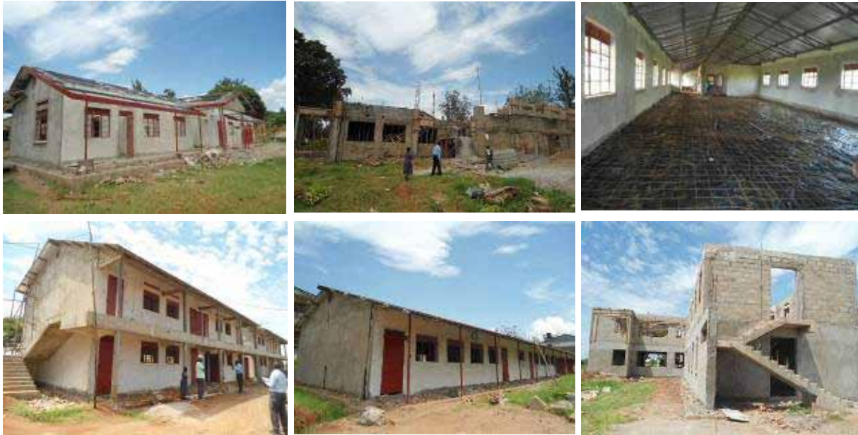
From the top left, the administration block at roofing level, the multi purpose hall, and the library block at finishes level From bottom left: the storied 8 classroom block at finishes, the sciences laboratory block at finishes and the storied dormitory block at roofing level at Tororo Girls
