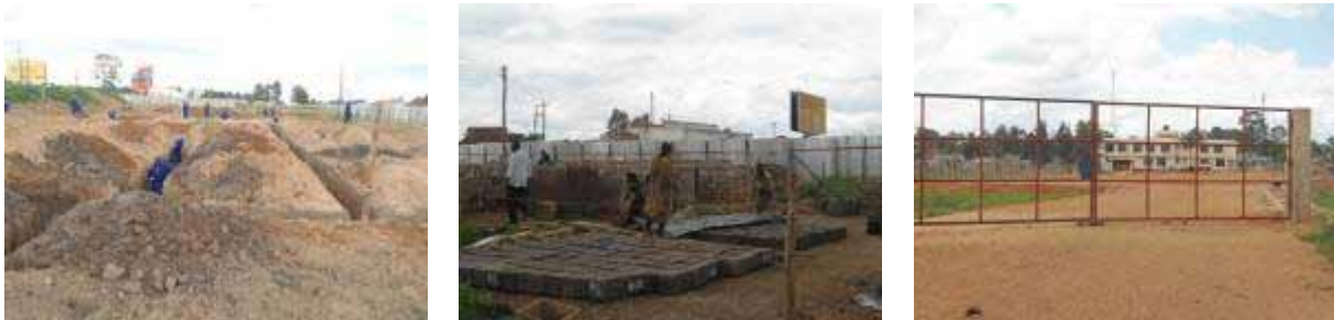
(Left); Excavation works at the site; (Centre); Making of blocks to be used for the construction works; (Right); A similar project to be synchronised Uganda's on the Tanzanian side that are almost complete
