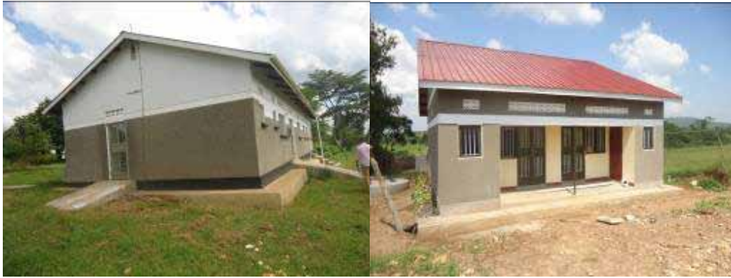
Construction of operating theatre at sekanyonyi HCIV and construction of a staff house at Kasikombe HCII Mityana district
