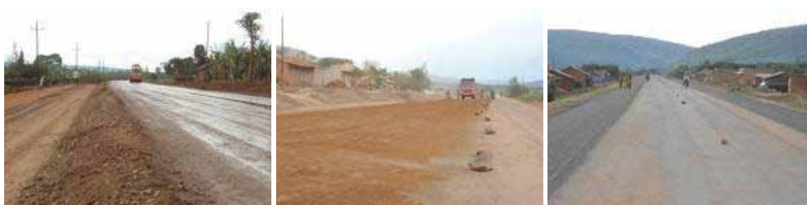
(Left): Ongoing base course works at Km 39+700; (Centre): Curing of a primed surface with sand at Km 46+980; (Right): Double surface dressing on the road shoulders and priming in the carriage way at km 49+931.
