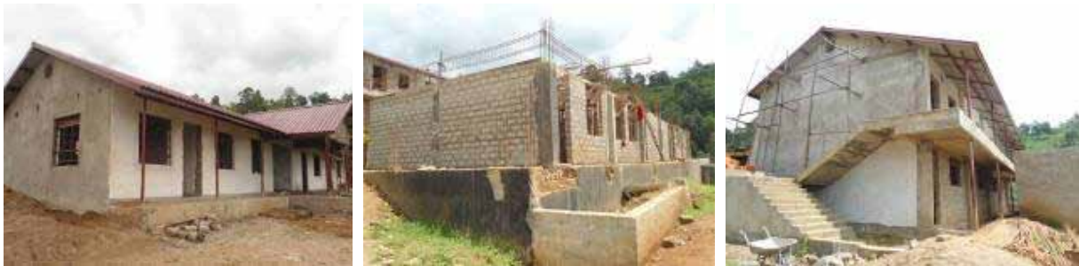
From left: The administration block at finishes level, the storied laboratory block at shuttering for the first floor slab and the storied multi purpose block at finishes level at Bumayoka seed school.
