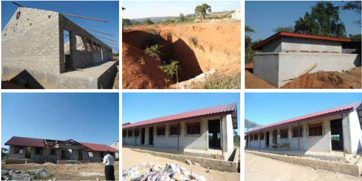
From top left: An administration block, 2 blocks of 2 classrooms each left incomplete From bottom left: A science laboratory at roofing level, a pit latrine behind the laboratory abandoned at excavation level and another VIP latrine left finishes level at Kalisizo S.S.
