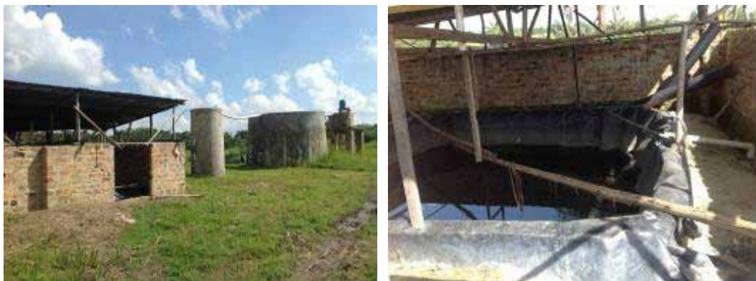
Water treatment system at Buloba Fish Farm
