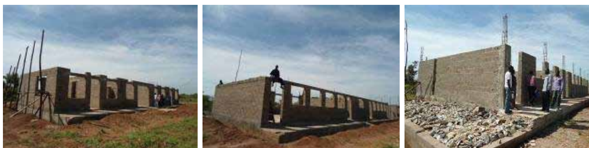
From left: The administration block and the 3 unit science block at ring beam level while the storied 6 classroom block they were beginning shuttering for the 1 st floor slab at Apo Seed S.S. Other structures were at the same level.
