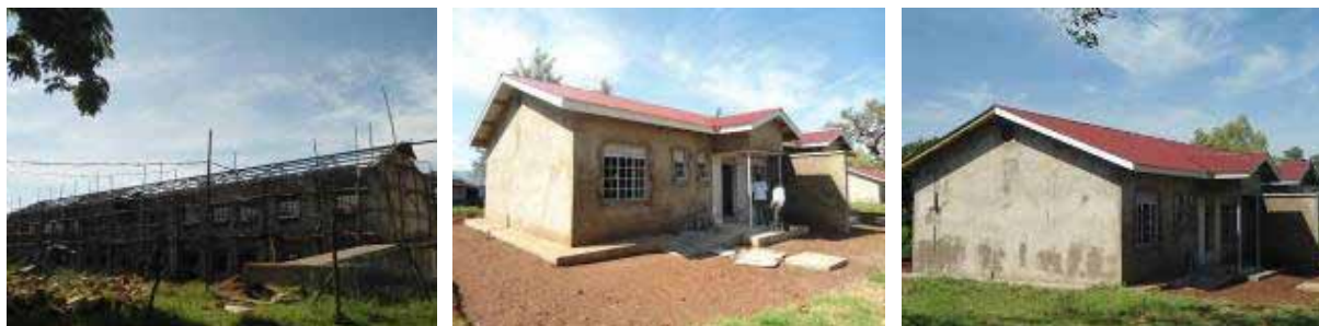
From left: The multi purpose block at roofing level, and 2 semi detached houses at finishes level at St Peter's College Tororo
