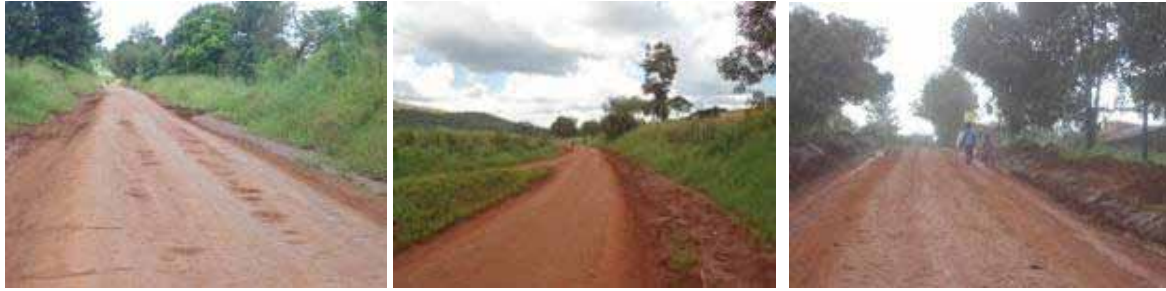
(Left): Damaged section due to poor drainage of Masindi-Kigumba road at Km 20+000; (centre); A graded section with high silt load on the right on Masindi-Hoima road; (right) A freshly graded section on Masindi-Biiso road at Km 26+500.
