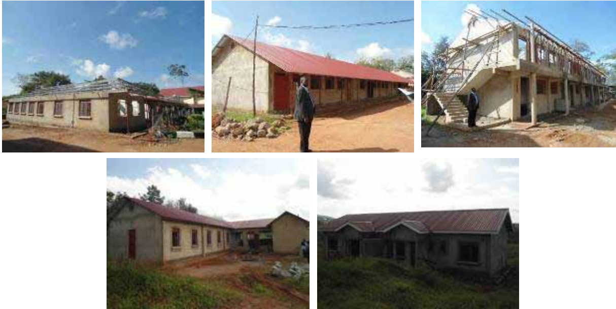
From the top left corner an administration block at roofing level, a 3 unit science laboratory, a storied 6 classroom block at roofing level From bottom left: a dormitory block at finishes level and a semi detached staff house at finishes level at Nabumali High School.
