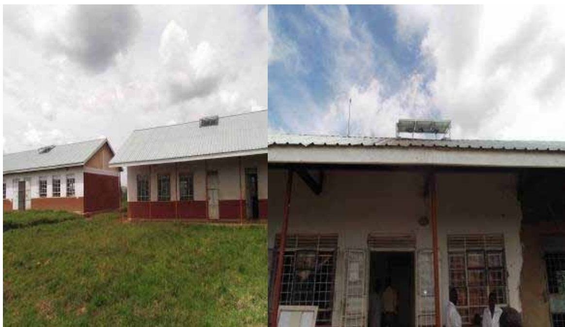
Installation of solar panels at Jangokoro Seed Secondary School and Ora Technical Institute Zombo district
