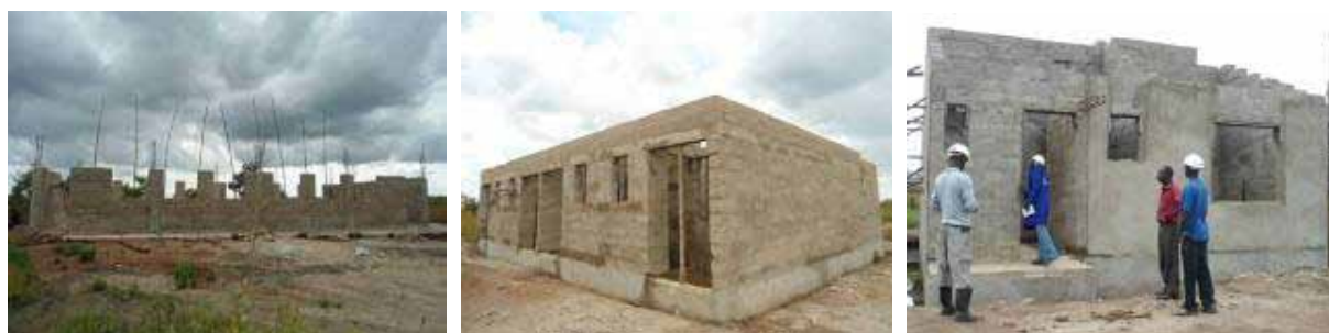
From left: The storied 4 classroom block going to first floor slab, a 4 unit teachers' house and the 2 bedroom house at wall plate level at Ramogi Seed S.S.
