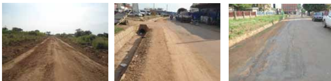
(Left): Bush clearing works for opening up of Kelin road; (Centre); Stabilised road edge awaiting priming along Market Street; (Right): Edge repairs on Jumabhai road.
