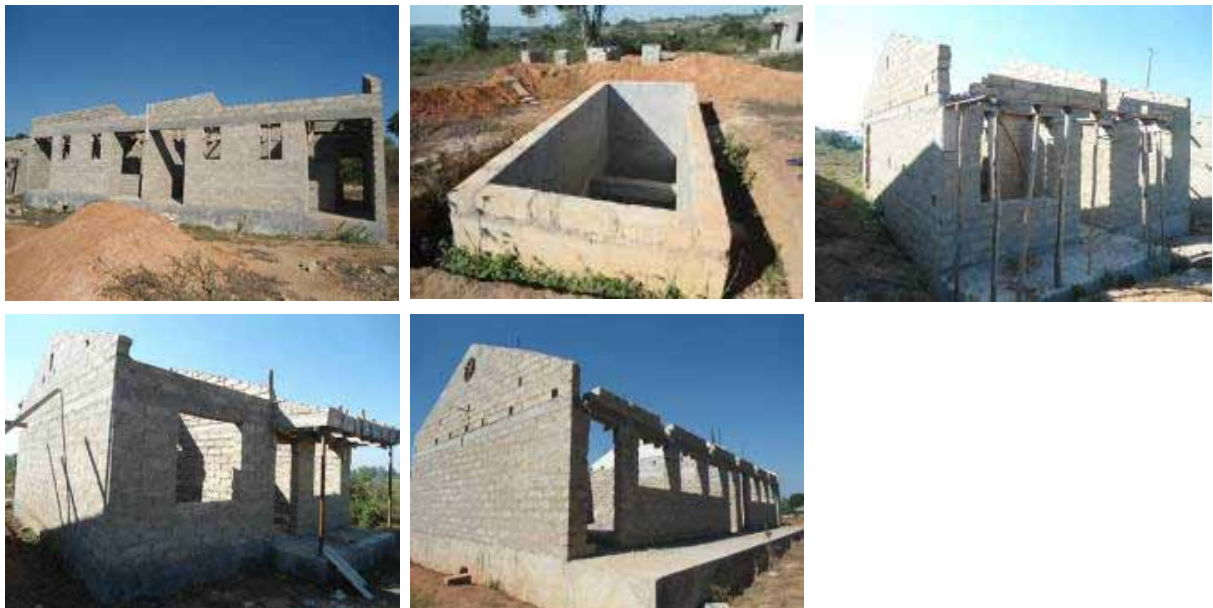
From the top left, A 4 unit teachers' house, a 5 stance VIP abandoned at slab level and a 2 bed roomed house, 2 bedroom housed abandoned at roofing level and another block abandoned at roofing level at Kalisizo S.S.
