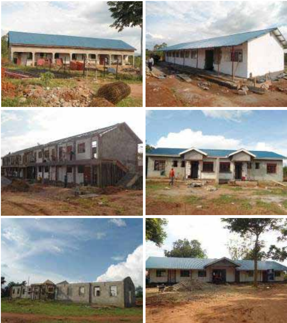
From the top left: The renovated boy's dormitory, a library and the storied six classroom block at roofing level. From bottom left: The semi-detached house at finishes level, a girls' dormitory at roofing level and the administration block at finishes level at Lumino High School.
