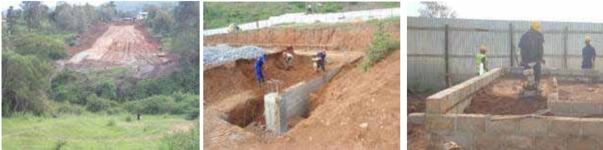
(Left): Road works ongoing on the Rwandan side but have yet commenced on the Uganda side; (Centre); Return, filling and ramming of soil into the excavations of the Customs and Immigration Block substructure; (Right) Compaction of murrum to make part of the floor of the Proposed Clearing Agents Building.
