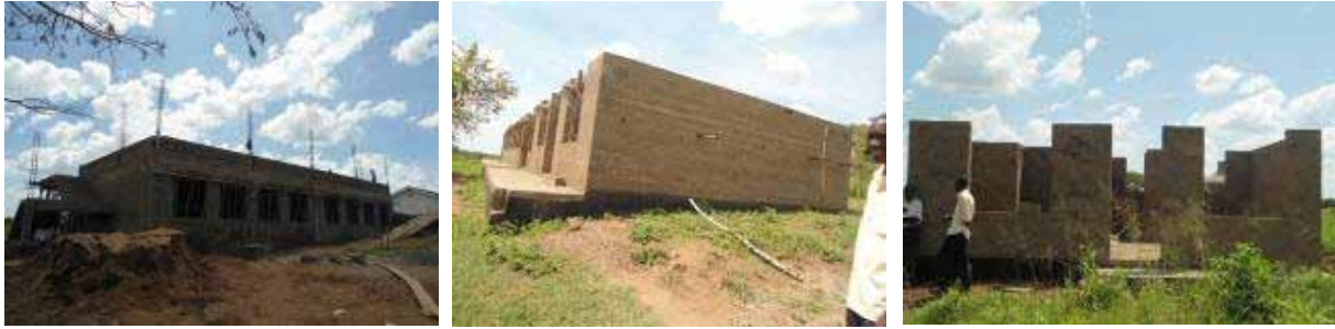
From left: The storied 4 classroom block at walling level for upper floor, the 160 seater library at ring beam level and the 2 bed room house at ring beam level a at Ayer Seed S.S.
