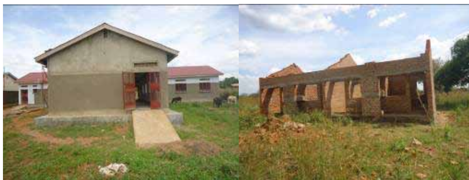
Construction of maternity ward Kitgum TC HCIII and stalled staff house at Lalekan HCII
