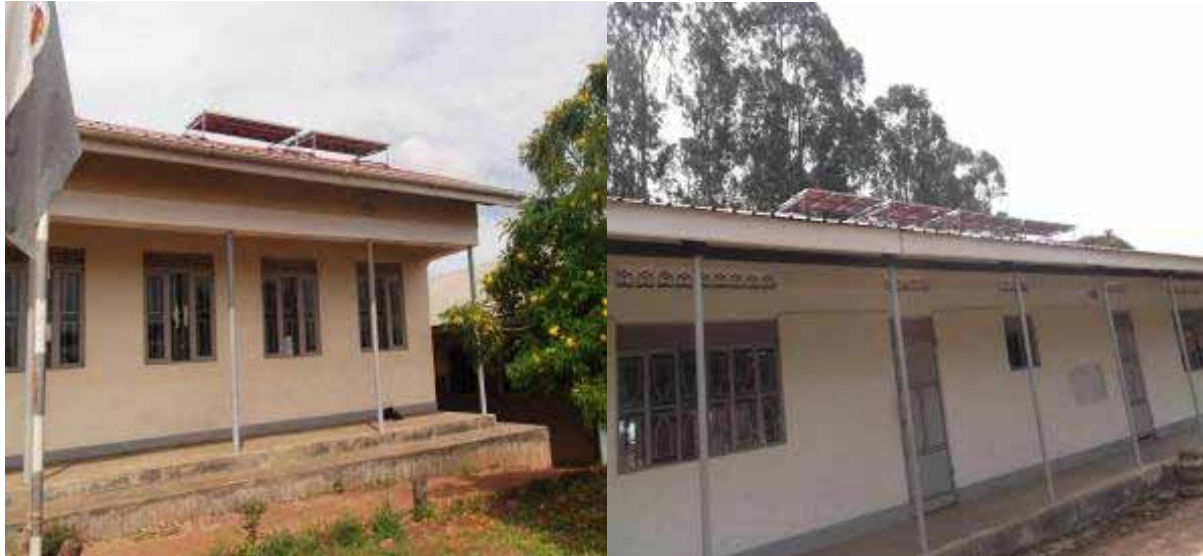
Solar Panel installation at Nyarilo Secondary School and St. Charles Lwanga Koboko
