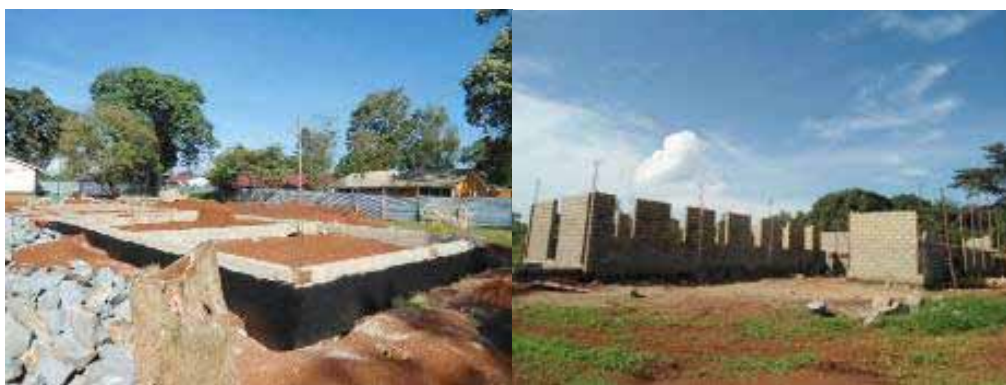
The administration block at ground slab level, while storied dormitory block under construction at Iganga S.S
