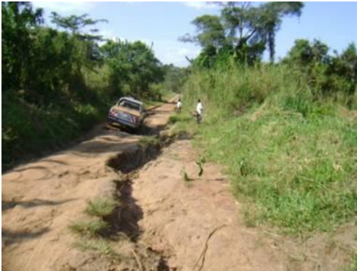
Example of a district road in Kibaale district which is beyond maintenance and requires rehabilitation.
