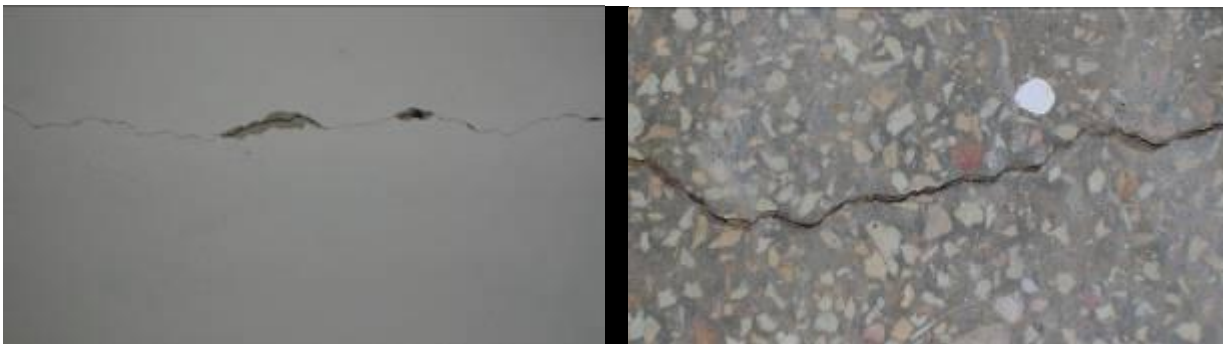
Cracks in a Theatre at Kamwezi HCIV,
