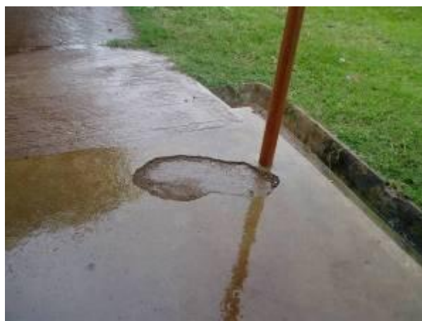
A cracked floor at newly constructed seed school at Bukedi S.S
