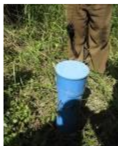
Failed drilling attempt 5 metres away from another failed site, by Kitgum DWO procured contractors, Dech Sub County, Kitgum
