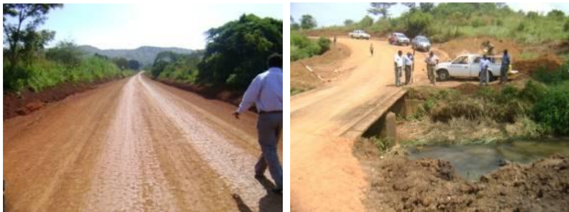
A finished section, and an existing timber bridge on Hoima – Kabaale - Kaiso road
