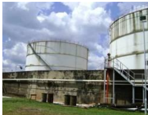
Dilapidated storage tanks
