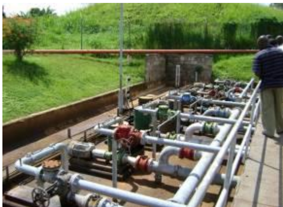
Some of the outlet pipes with leakages
