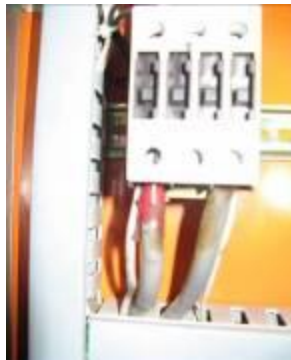
Broken fuse still not fixed by the contractor , at Delo pump house, Yumbe
