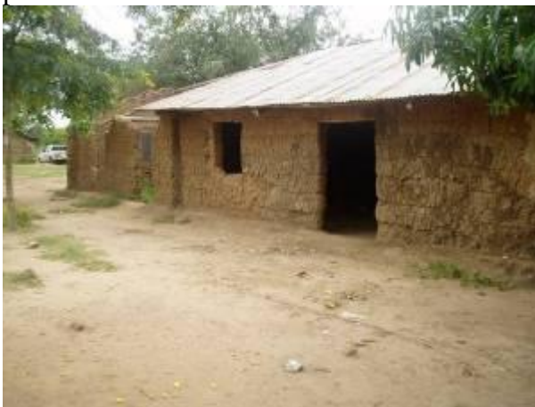
Part of the classroom block that had collapsed
