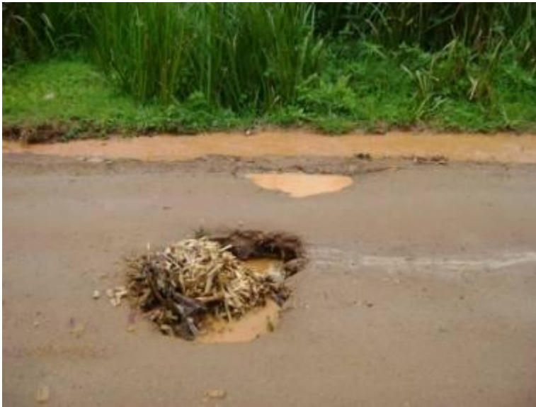
A collapsed culvert on a road recently maintained using force account in Bushenyi district
