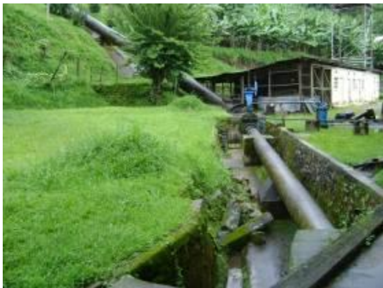
Penstock for Mobuku power plant (Kilembe)
