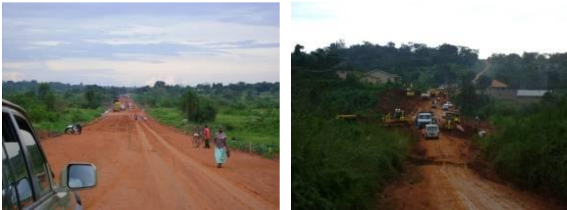
A newly filled swamp and ongoing earthworks on Kampala – Gayaza – Ziobwe road
