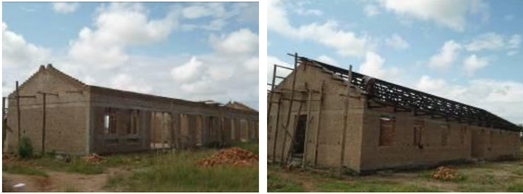
The twin workshop and the dormitory at roofing level at Wera TS
