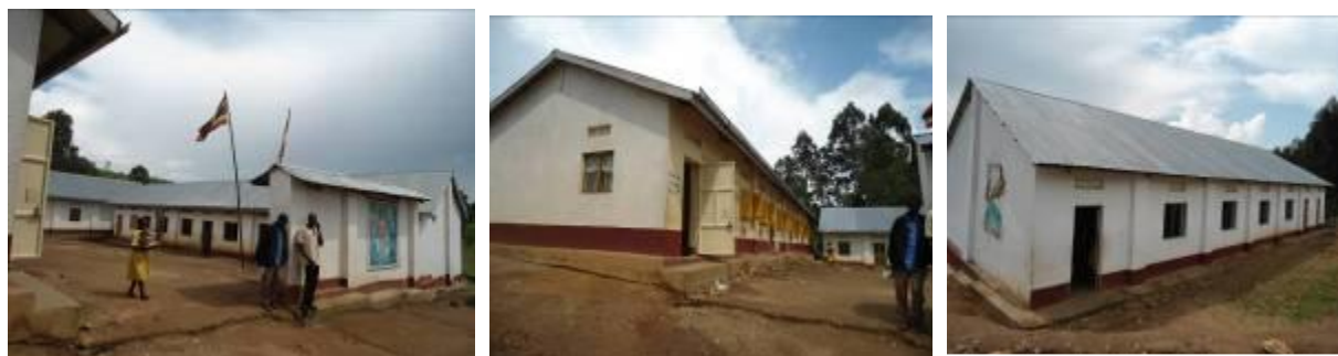
Some of the structures on the purchased land: the ten classrooms, the main hall and a five classroom block with an office
