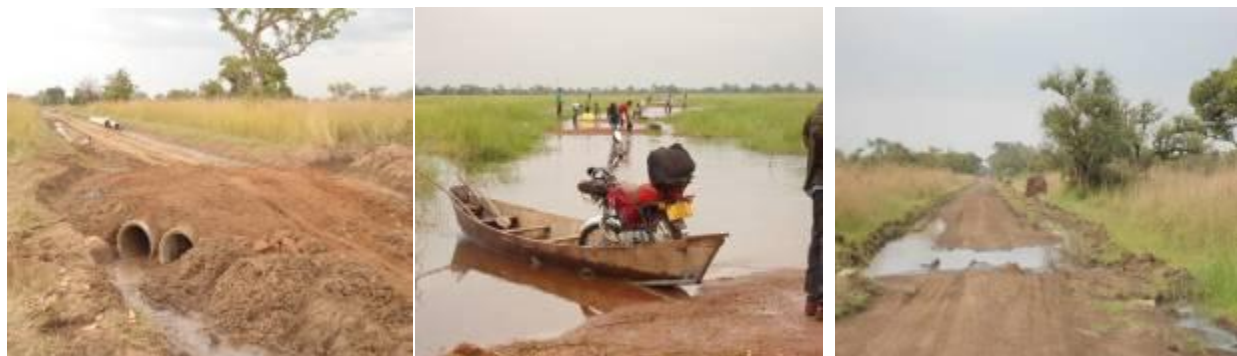
Sections of Soroti-Gweri-Kapujan-Toroma-Magoro-Ngariam (Left): Double culvert installation works at km 1+000 from Ngariam. (Centre): Drainage problem due to flat terrain at Km 13+000 from Ngariam. (Right): well graded and gravelled section in good condition at Km 5+800 from Soroti-Mbale road. Note the slashing done by the LBCs. Further ahead is the 6Km swamp had submerged the road.
