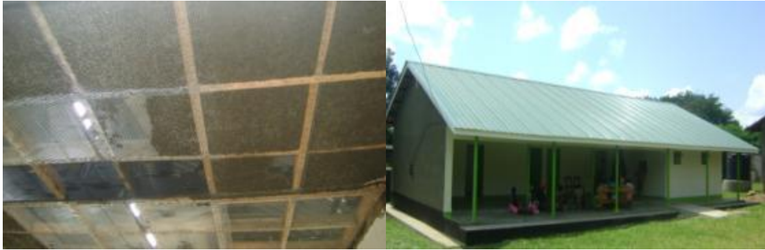
Mbale Local District: ceiling of maternity ward at Bumadanda HCIII (left); OPD at Lwangoli HCIII (right)
