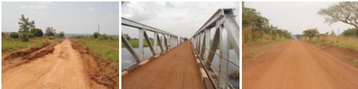
Left); Section of Arapai-Katakwi road showing deterioration at Km 15+100. (Centre); Komolo bridge works along Arapai-Katakwi road at Km 29+300 showing the new kerbs and sprayed guard rails. (Right); Section of Katakwi-Iriri at showing a well graded and gravelled road still in good condition
