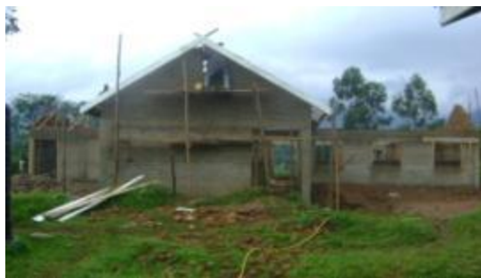
Kabarole District PHC Development: construction of a general ward at Kisomoro HCIII (above)
