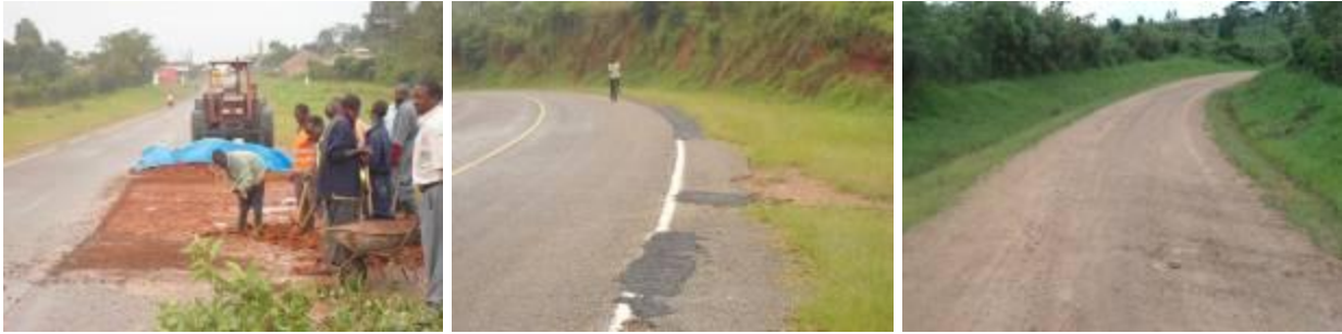
(Left); Ongoing gravel and asphalt patch works along Mabara-Ibanda road at Km 22+700. (Centre): Asphalt patches at the edges at Km41+600 along Mbarara-Ibanda road. (Right); well graded section along Muzizi-Buremba road in good condition
