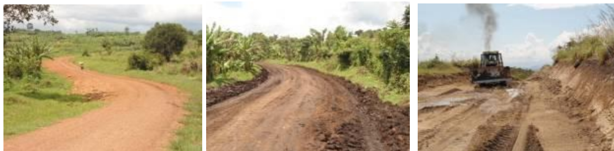
Sections of Kamwenge-Dura-Rwimi road (left) completed graded and gravelled section still in good condition; (centre); a section that had just been graded; (right) cutting to spoil aimed at widening of the road at a narrow section.
