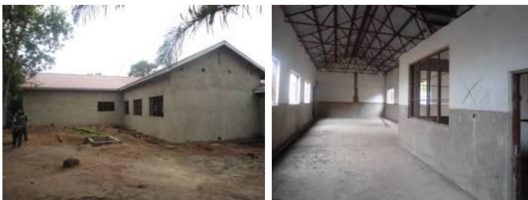
Side view and internal works of the fruit juice processing plant in Arua
