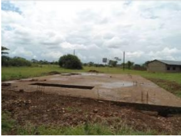
The poorly done slab for the MV workshop at Iyolwa TS
