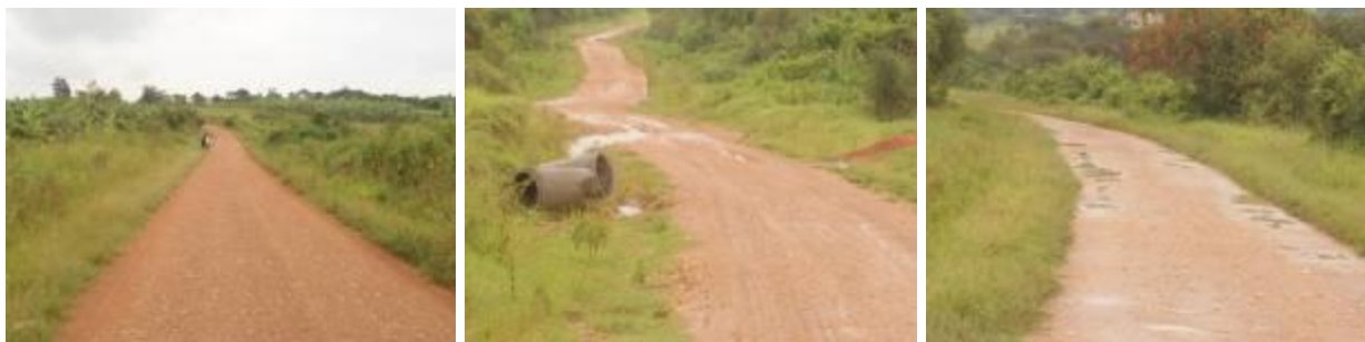
Sections of Biharwe Bwizibwera road (Left): Km2+000 with a good running surface. (Centre); Km14+100 where culverts were yet to be installed with water crossing on top of the road. (Right): Km19+100 developing potholes which are likely to damage the road sub grade
