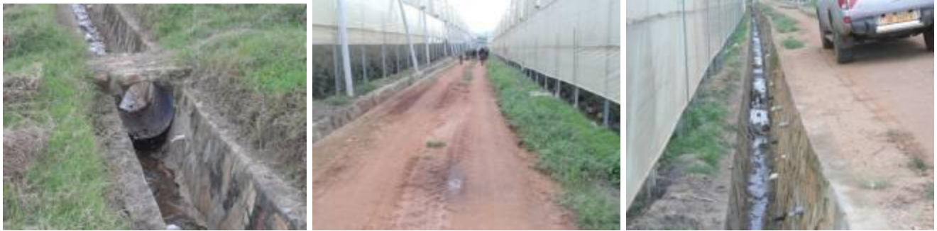
Left); Drainage channel with stone pitching and culverts works. Centre); The 0.86Km, 5m wide road that was graded and gravelled. Right; Retaining wall about 1.5m along the 0.86Km access road.
