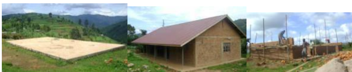
Kabale District PHC Development: foundations of OPD at Shebeya HCII (left); OPD at Kitanga HCII (centre); construction of staff houses at Kahama HCII
