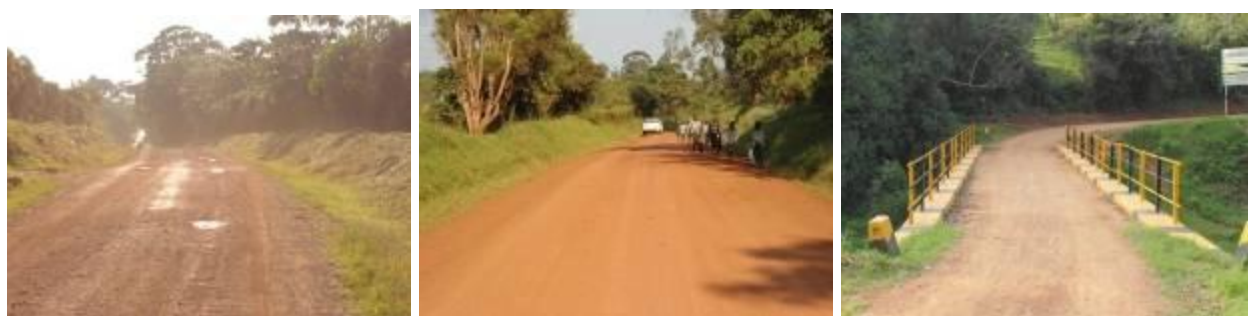
Sections of Fort Portal-Kijura road (left) graded section of the road developing potholes; (centre); spot gravelled section still in good condition; (right) Sogahe bridge at the end of the road..
