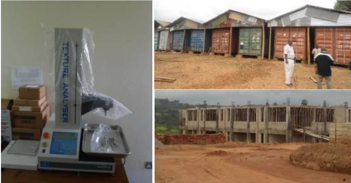
Installed analyser, delivered equipment in containers and stalled construction of quality control laboratory block
