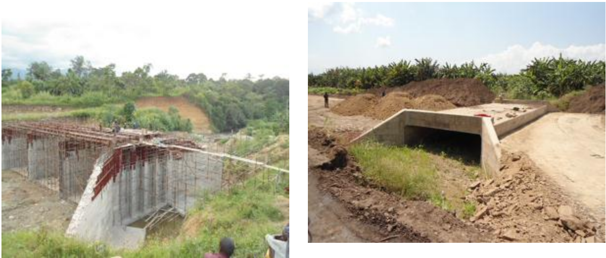
Fort Portal-Bundibugyo-Lamia road; (left) Ndugutu bridgeworks at Km 100+950c; (right) one of the box culvert installation
