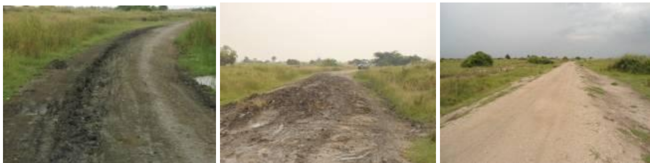
Sections of Rwebisengo-Rwangara road (left); at Km1+500 – depressed wheel tracks (centre); at Km9+000 where the road is almost impassable. (right); at Km21+100 – one of the well graded and gravelled sections
