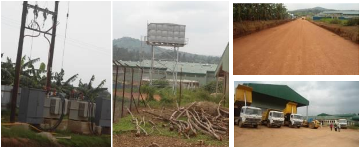
Installed transformers and Water tank; graveled road and parked trucks at Nyaruzinga
