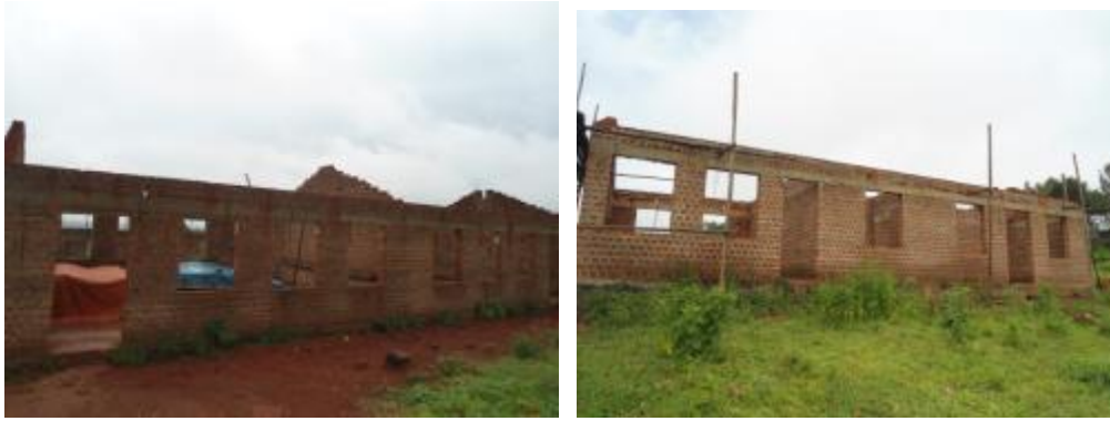
A two classroom block and an administration block at wall plate level at Burunga S.S.
