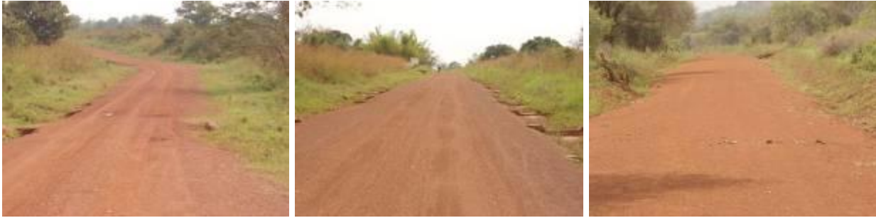
Sections of Kitgum-Orom road (Left); Km 18+400-road is being eroded and developing potholes. (Centre); Scour checks at Km 22+200 constructed along the sides of the road reduce on erosion. (Right); well graded and gravelled section still in good condition at Km88+800.
