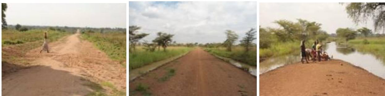
Sections of Amuria-Acowa-Usuk (Left): Sandy section undergoing silting and erosion between Km 0+800 and 1+500. (Centre); Well graded and gravelled section still in good condition with water at the road sided due to the fl at terrain. (Right); Inaccessible road after Km 8+500 at Ajelek Swamp
