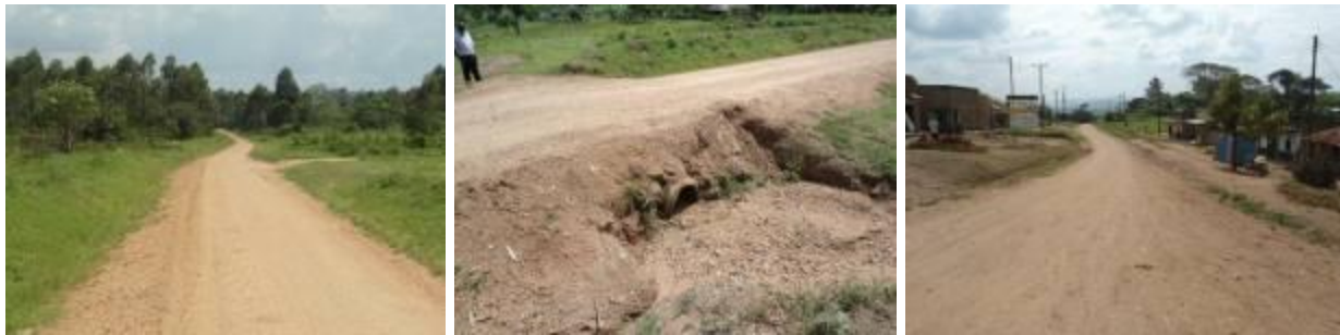
Sections of Ishongororo-Bishese road (Left); Km2+200 showing re-gravelled works with a good running surface. (Centre); Km16+700 showing a culvert line with no headwall about to be blocked due to silting. (Right); Km22+700 showing a graded road surface at Ishongororo Trading centre.
