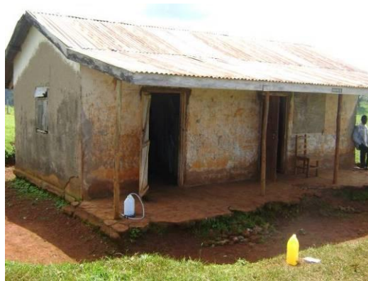
Dilapidated office building
