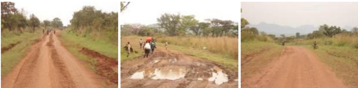
Sections of Orom-Locomo-Karenga road (Left and Centre); Graded sections undergoing major deterioration due to drainage problems that were yet to be fixed by the client. (Right); graded section at Km 17+400 still in good condition with LBC routine maintenance works done on the sides of the road.
