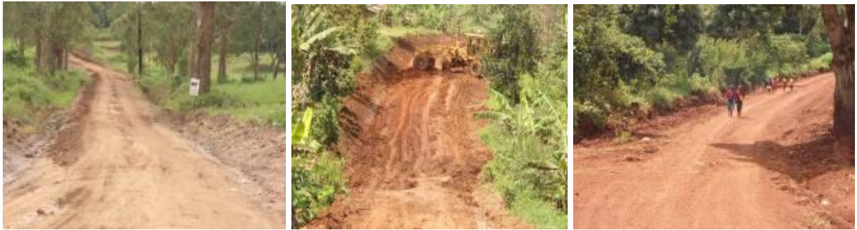
Sections of Mikka-Buwembo-Kitayita road - grading activities, (left); at Km0+000 (centre); at Km7+300 (right); at Km14+100.
