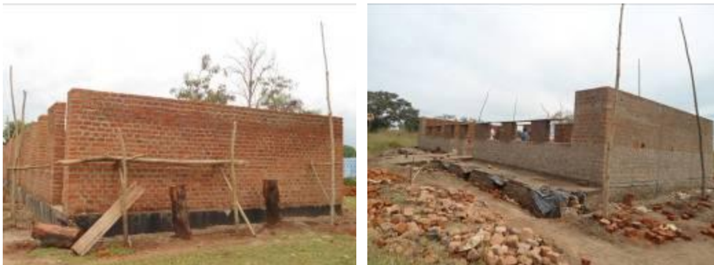
The three classroom block and the twin workshop at ringbim and walling levels respectively at Kumi TS
