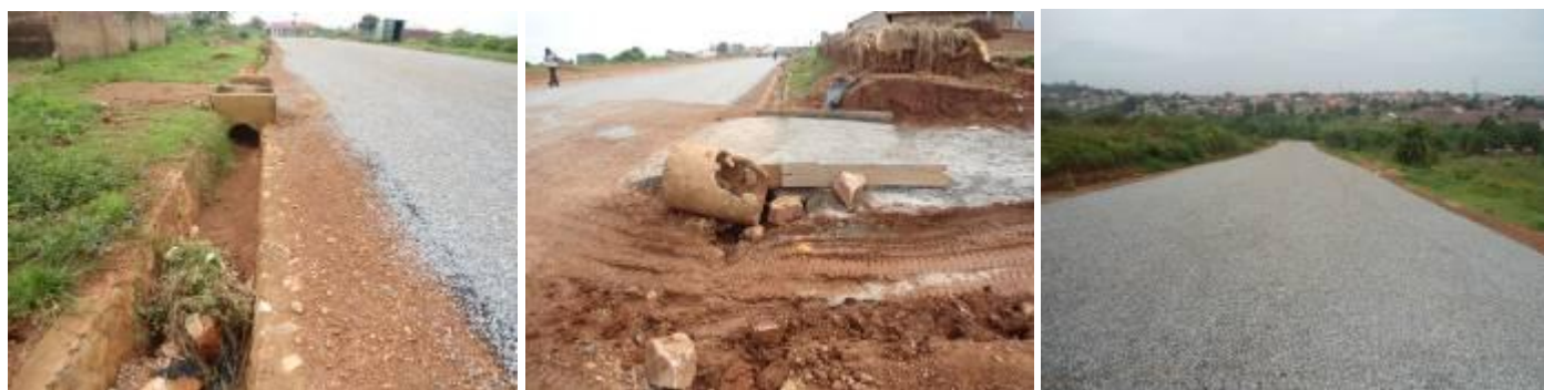
L-R, Unsealed shoulders, broken culvert and a sealed section of First Street
