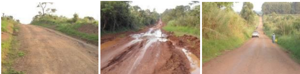
Sections of Sogahe-Kyarusenzi road (left) graded section at KM 12+800 with deteriorated surface due to lack of drainage structures; (centre); a section where water is crossing on the road surface; (right) graded section of the road in good condition.
