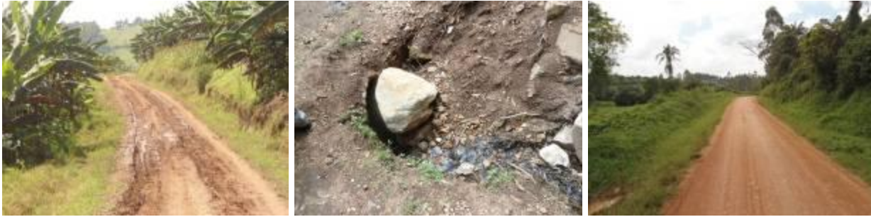
Sections Kyankanda-Bitsya-Ruhoko road (Left): Km2+900 showing muddy and rutting wheel trucks. (Centre): Km16+300 showing a culvert blocked by a boulder due to landslides. (Right); Km36+000 showing a well graded and gravelled section still in good condition.
