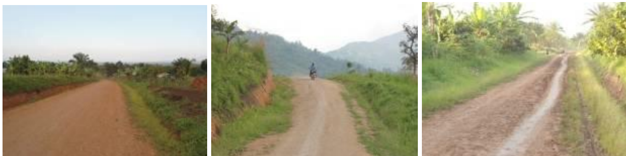
(left) completed graded and gravelled section in good condition; (centre); a graded; (right) section of Bubandi-Bundibugyo Army Barracks-Butama Health Centre road which is deteriorating due to poor compaction and no gravelling.
