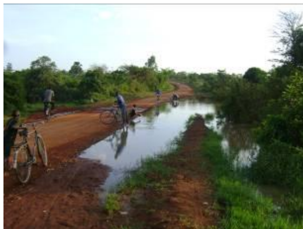
Ngeta – Kitgum Bdr road: water crossing and almost cutting off graveled section of the road
