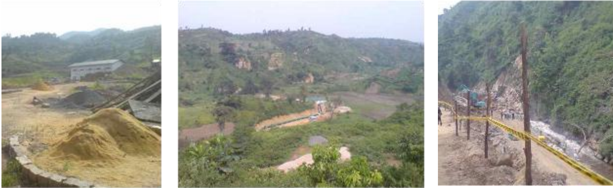
Ishasha hydro-electric plant: powerhouse (front view); penstock pipes (aerial view); weir construction.
