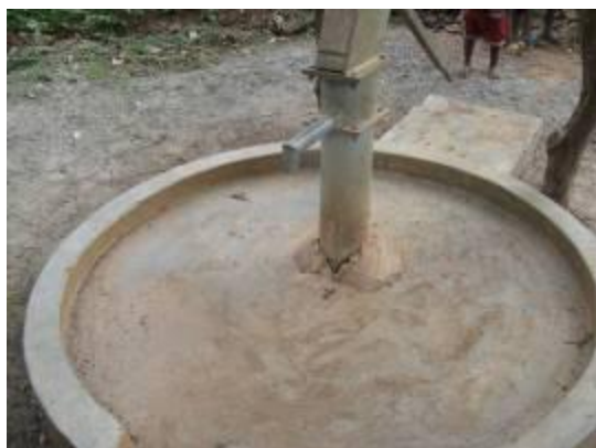
Poor quality works and non functioning borehole, Wakiso district
