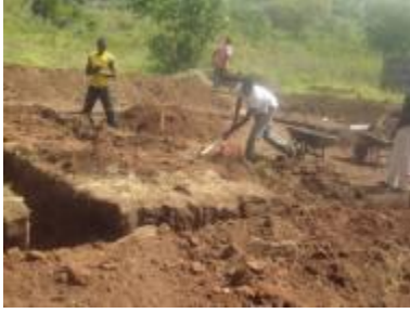
THE FOUNDATION FOR THE 4 CLASSROOM BLOCK BEING EXCAVATED AT ST. CHARLES LWANGA S.S. KALONGO
