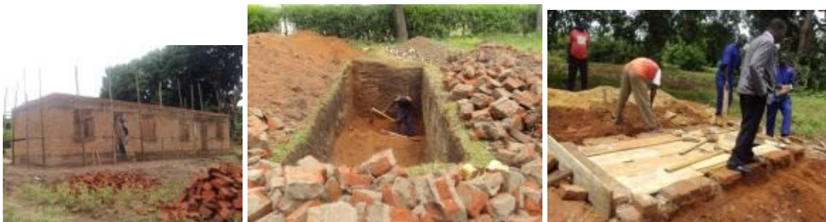
The semi detached house, 2 stance pit latrine for staff, and the 4 stance pit latrine for the students at Ngora High School
