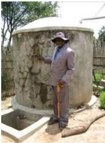
Beneficiary pointing to leakages, Shuuku sub-county, Bushenyi district
