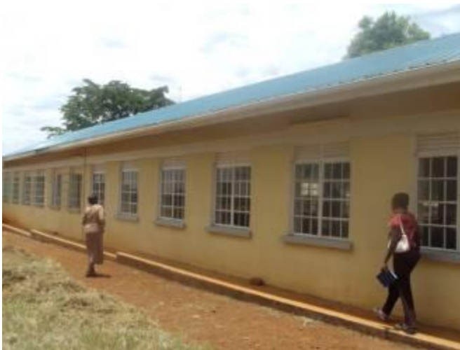
The Principal taking the monitoring officer around the building with defects
