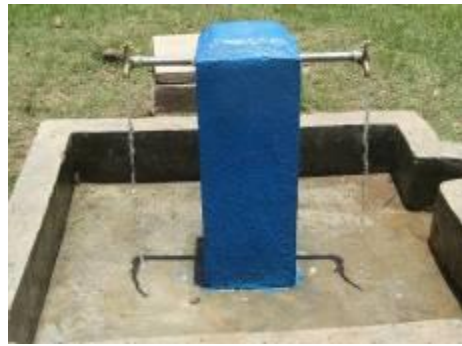
Water flowing in Ombatini Secondary School, Wandu, Maracha Terego district
