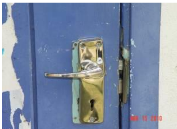
Arua Telecentre entry locked tampered with during an attempted break in
