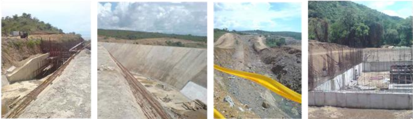
Buseruka hydro-electric plant: construction of forebay; complete section of power channel; incomplete approach channel; construction of powerhouse.
