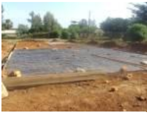
The sub-structure for the dormitory block being casted at Madera School of the Blind
