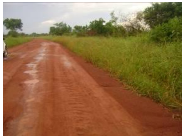
Gulu - Aswa road: impending failure of a graded section of the road.
