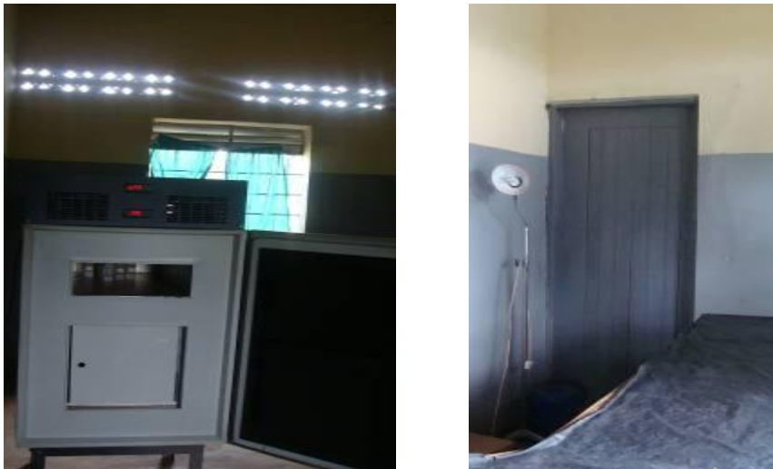
Solar fridge, and lamp in Health units.
