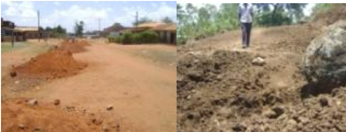
Pictures show ongoing works on Namunsi – Nakaloke – Kaloyi and Mulatsi – Busoba roads in Mbale district.
