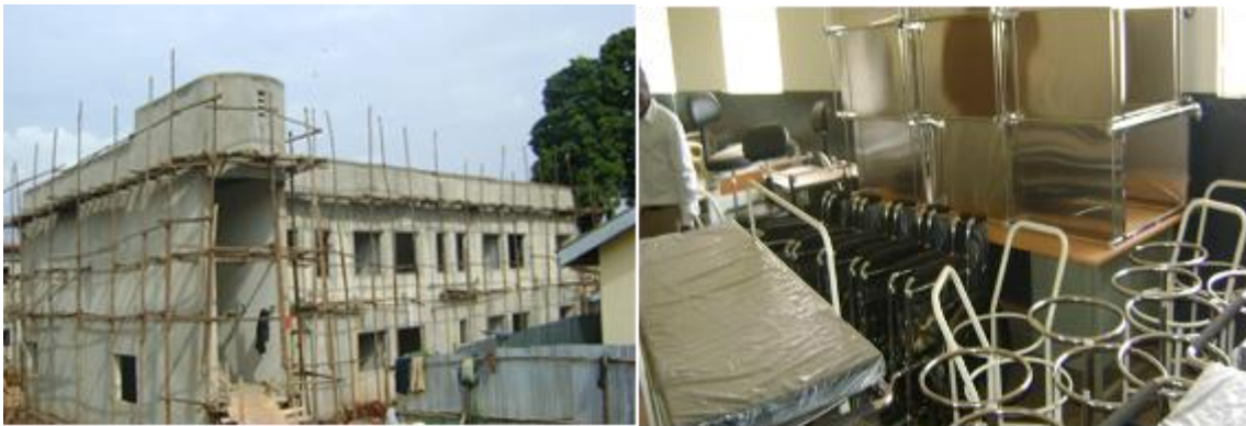
Jinja Regional Referral Hospital; construction of the private ward (left) and new medical equipment (right)
