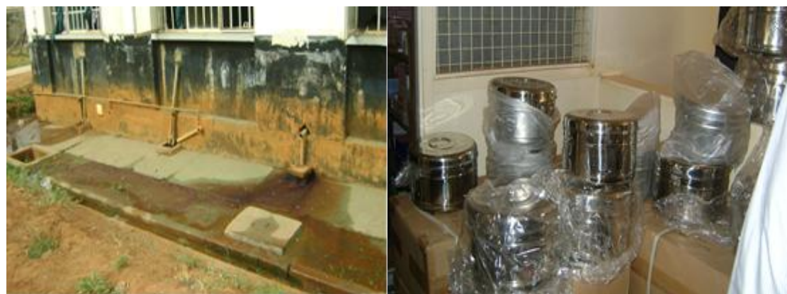
Gulu Regional Referral Hospital; blocked sewer line under renovation (left) and medical equipment that was supplied (right)
