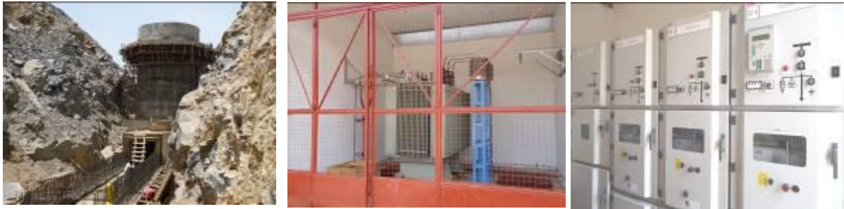
L-R: Surge shaft under construction, Installed Generation transformer and Switch board at Nyagak Hydro Power
