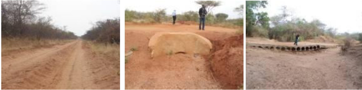
Sections of Lokitanyala – Loro – Amudat Road (48.6Km) at 3+200 (Sandy soils and road below surrounding ground), 7+200 (Silted culvert crossing likely to have collapsed will eventually make the road impassable if not attended to) and 22+300 (Existing drift has been eroded and undermined by storm water).
