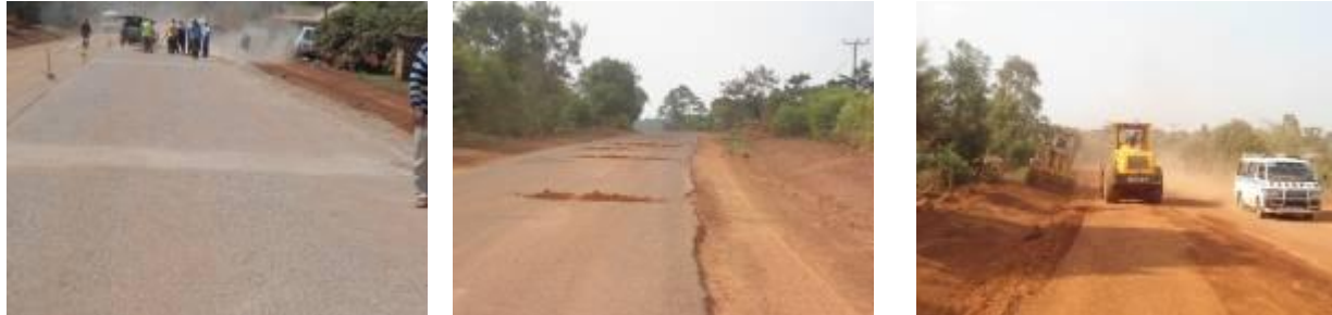
(Left); Trial section of 450m being prepared for priming (Centre); Existing section of the road that is being maintained. Note the potholes that are being filled with murram to make the section motorable. (Right); A section undergoing benching works of the foundation.
