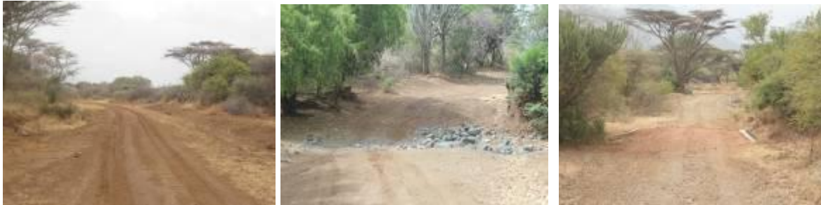
Sections of Katekile – Tapach Road (11Km) at 5+100 (graded with cattle Track to the left), 5+800 (River Crossing that requires construction of drift) and 7+900 (Newly installed culvert Crossing).
