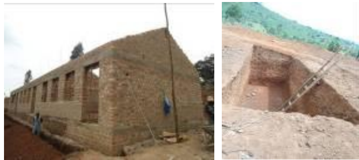
A 3 classroom block at roofing level and a 5 stance pit latrine at excavation level at Karera T/I
