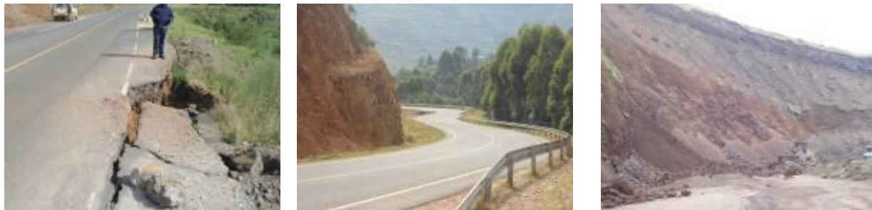
(Left); Completed section of the road whose edges are flaking off necessitating shifting of the road inward. (Centre): Completed section that has been handed over to the client with road markings and road furniture. Notice how the terrain is affecting the project path. (Right); Some of the sections where clearing and grubbing is still ongoing that is aimed at shifting the road inward to avoid failures like in the picture on the left.
