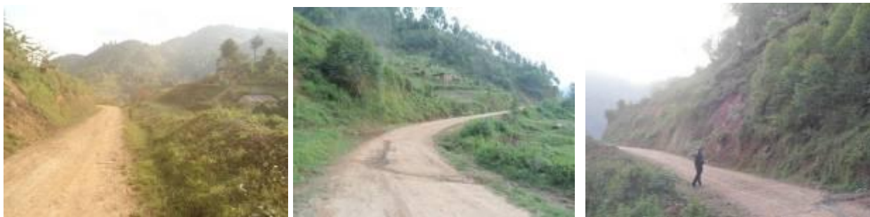
Sections of Kisoro – Nyabwishenya – Nteko road; (left) ; a well graded section in fairly good condition; (centre); a deteriorating section caused by water running on the road surface; (right) a section prone to landslides due to nature of soils and the agricultural activity.
