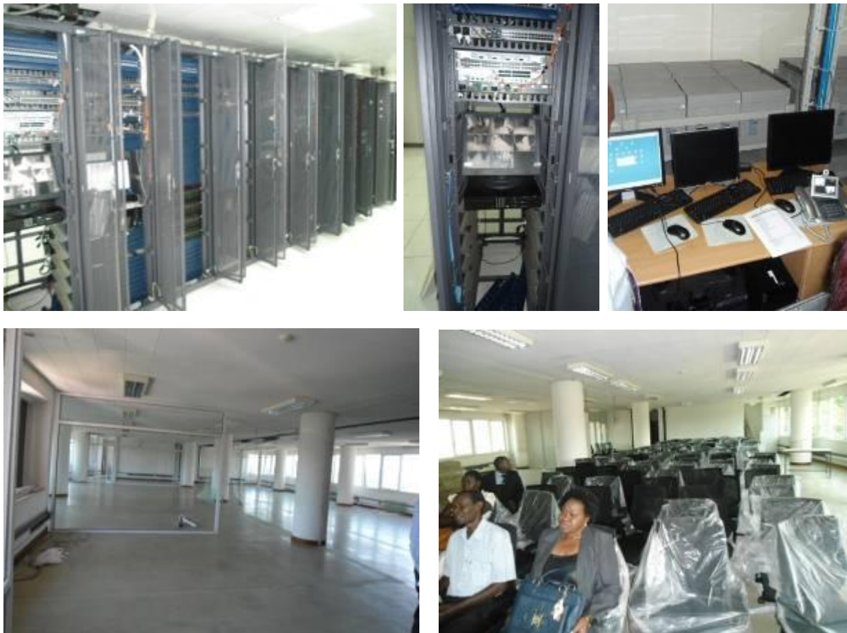
Top: Mounted BPO Servers, Security monitoring display, Server work area; Below: Partitioned BPO incubation centre on 3 rd floor and delivered furniture on 4 th Floor of Statistics House
