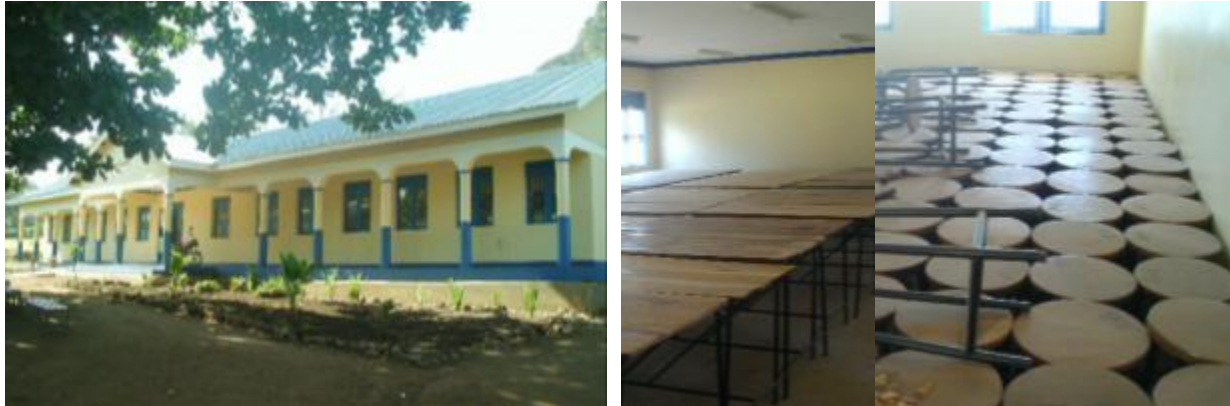
Front view of ICT lab, completed ceiling and delivered furniture at Rock High -Tororo
