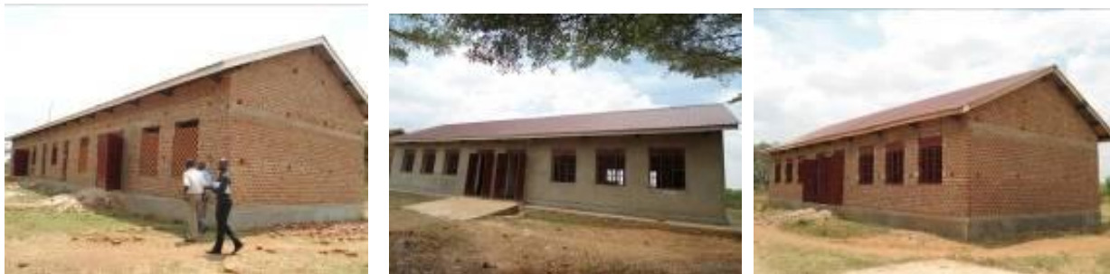
The 2 blocks of classrooms and a twin workshop constructed at Nagwere T/I
