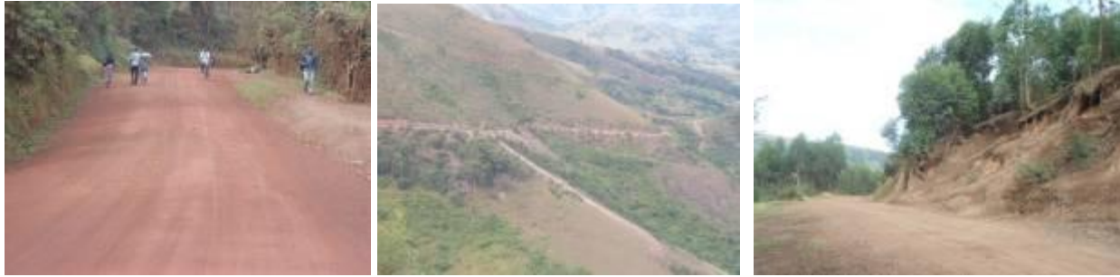
Sections of Butobere – Muyubu – Rwamucucu road; (left) ; a well graded and re-gravelled section in good condition; (centre); the terrain in which the road traverses that affects the manoeuvring of construction equipment ; (right) a section prone to landslides resulting from rock mining from road embankment.
