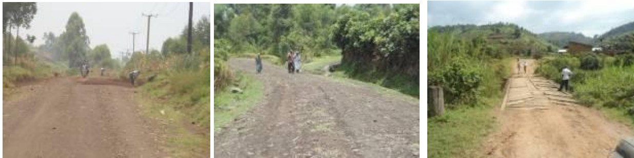
(Left); Section of Kisoro-Kyanika road with LBC works of back sloping and clearing of side drains; (Centre); Section of Kisoro-Nyarushiza-Muhabura road with protruding rocks that require specialised equipment for maintenance which the station lacks; (Right); A wooden bridge over Kaku river on Natete-Busanza road that requires replacement.
