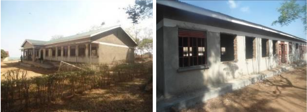
Front view of the near complete ICT lab and hind view showing missing windows and gutters at Wanyange Girls' SS
