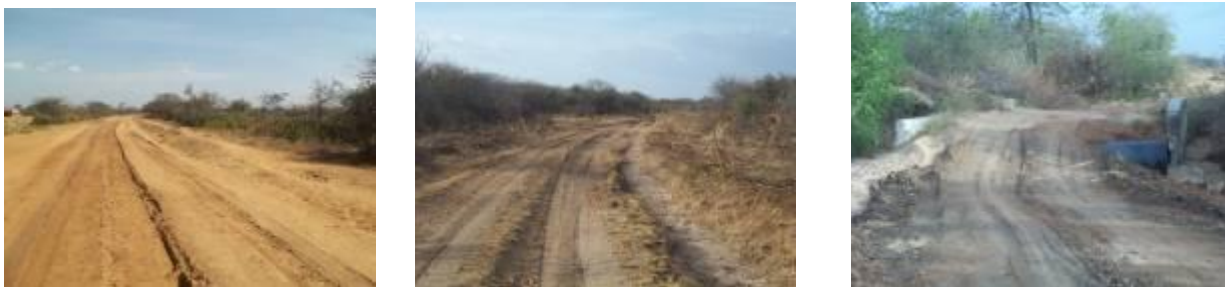
Sections of Amudat – Kalita Road (66Km) at 4+700 (Gullies along the road due to failure if the drainage structures to accommodate the runoff), 26+700 (Bush clearing in progress) and 28+100 (Stream crossing with culverts exposed)
