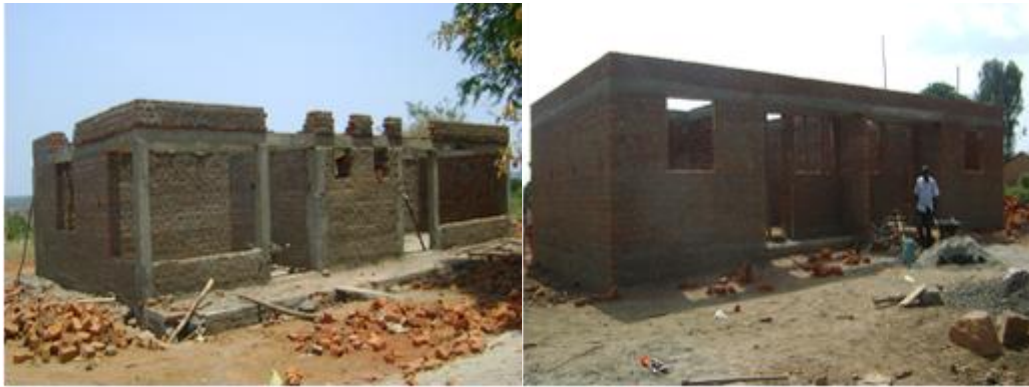
Arua District Local Government; OPD/maternity ward at Ogoko HCIII (left) and semi detach staff house at Aroi HCIII(right)
