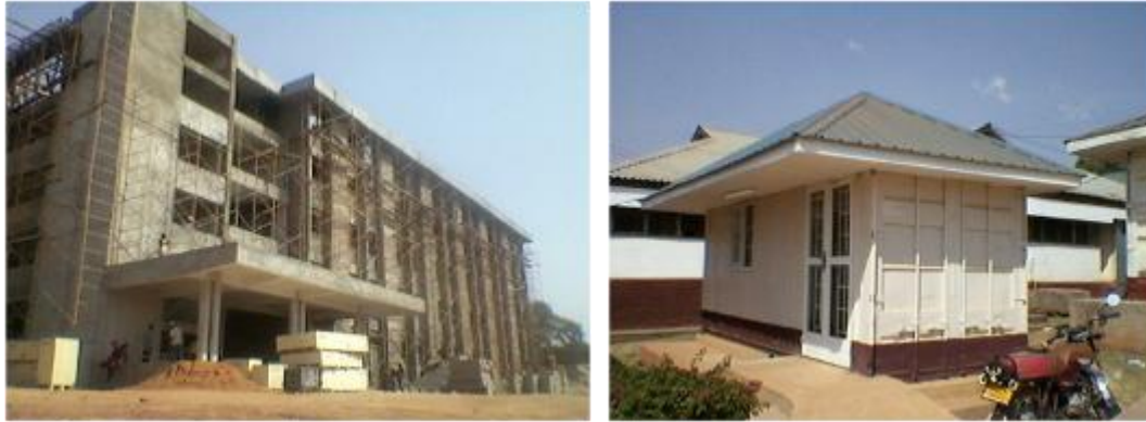
Uganda Cancer Institute; new cancer ward (left) and remodeled container into drug stores (right)
