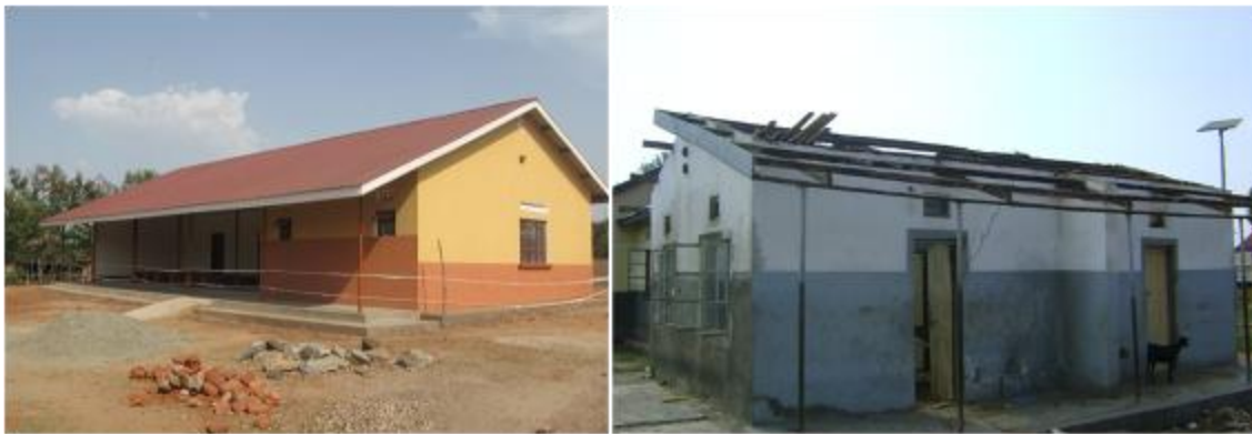
Nebbi District Local Government; OPD near completion at Pacego HCII (left) and rehabilitation works on staff house at Pakwach HCIV (right)
