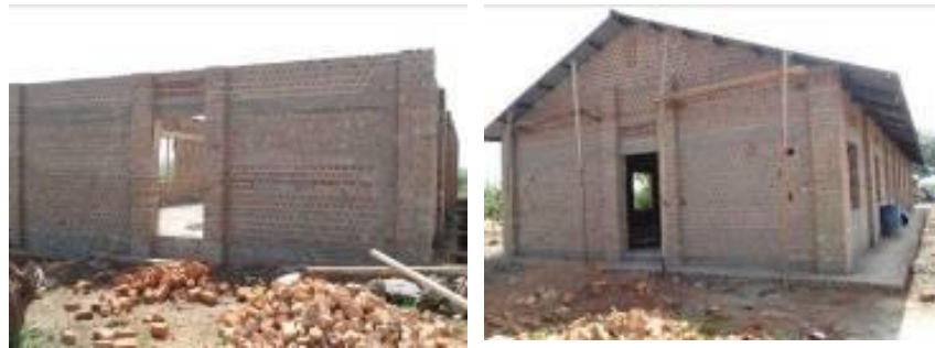
A boys' dormitory at wall-plate level and a girls' dormitory at finishes level at Ngoma S.S
