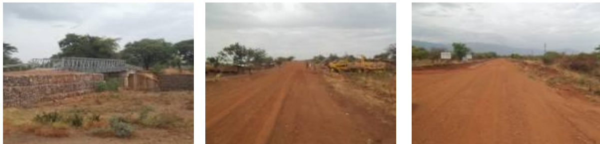
Lorengedwat Bridge and Sections of Lokapel – Chosan Road (33.5Km) at 22+400 (Graded road but not compacted with the station equipment parked due to lack of tyres) and 33+500 (graded and compacted section at Chosan)
