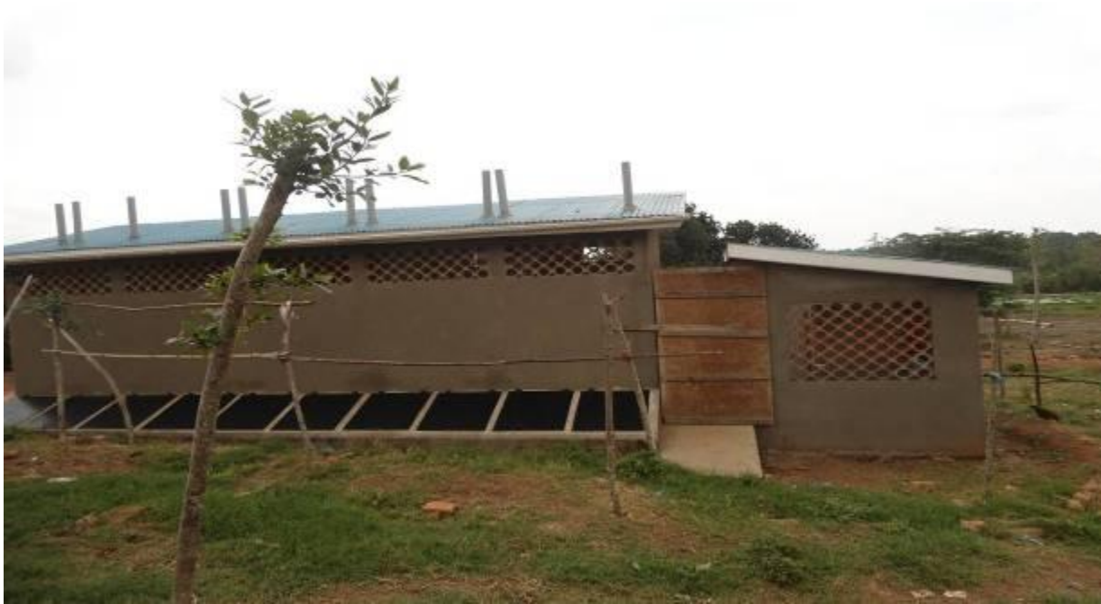
Public VIP ECOSAN toilets built at a market place as part of Nakaseke Town Piped Water Supply Project. Over six months since its completion, it is still sealed off and unused. (07/03/2012)
