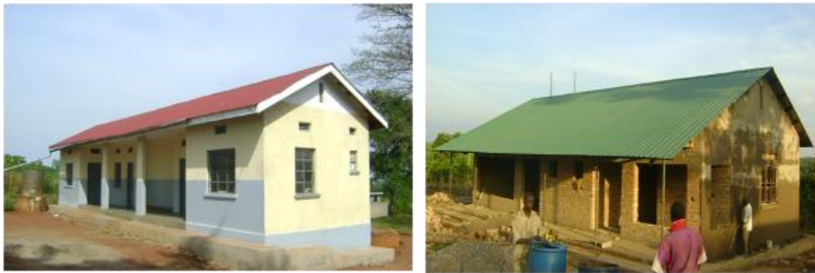
Sembabule District Local Government; partially renovated staff quarters at Makoole HCII (left) and OPD construction at Kayunga HCII (right).
