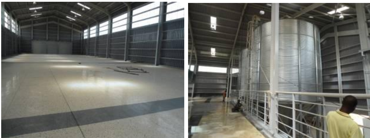
Polished floor of the main processing plant and final touches on the installed silos
