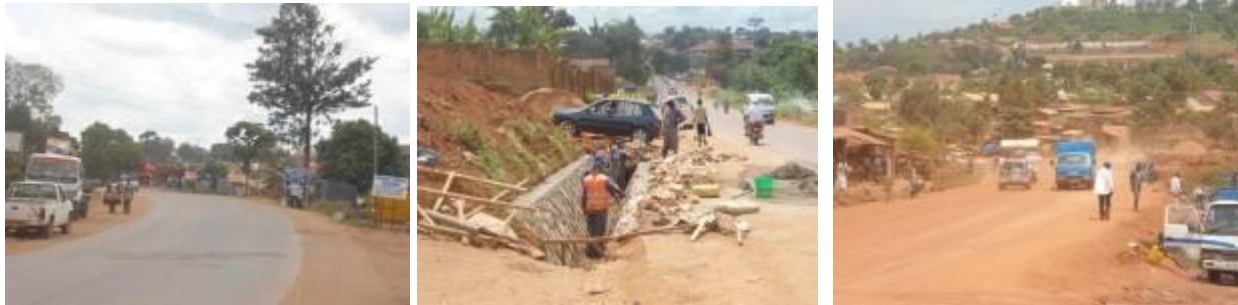
(Left): Completed section of Kireka-Namugongo road showing part of the wearing course that was destroyed by fire during riots; (centre); Drainage works ongoing near the Namugongo trading centre; (right) The 300m of Silver Springs-Bweyogere at Kinawataka junction that is at the formation level.
