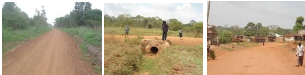
Sections of Nazigo-Kireku-Nkokonjeru-Kitimbwa Road (left) completed graded and gravelled section still in good condition; (centre); a newly installed 600mm diameter culvert line at 11+400 from Kitimbwa Trading Centre near Nongo Town. ; (right) a section toward the end of the road that is beginning to deteriorate with potholes due to heavy traffic.
