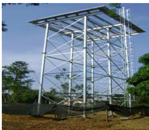
Arua Regional Referral Hospital; water tank (above)
