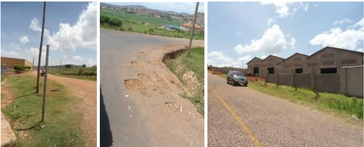
Vandalised road signage, potholes developing on completed section and new factory under construction in Luzira industrial park
